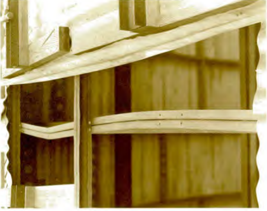
Figure 11. Top view of one of the ribs shown in Figure 10. The sheeting was removed to take picture.
