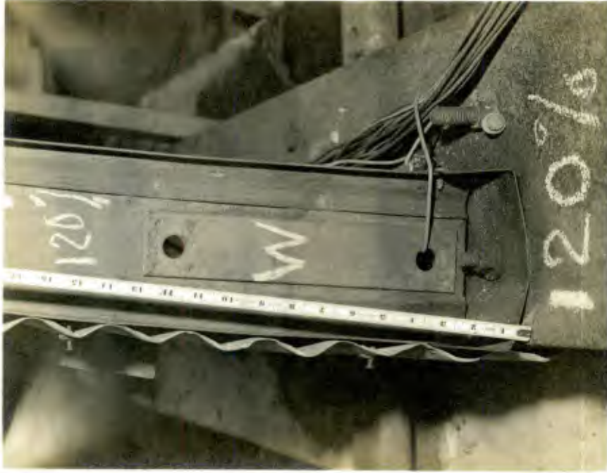
Figure 12. Base shoe pulled 1/2-in. away from foundation at 120% of wind load.
