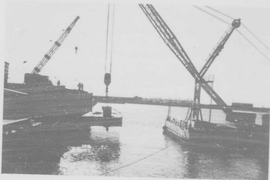
Figure 17. 3 x 12 ramp barge about to be launched from nearly horizontal position (11-ft rail height).
