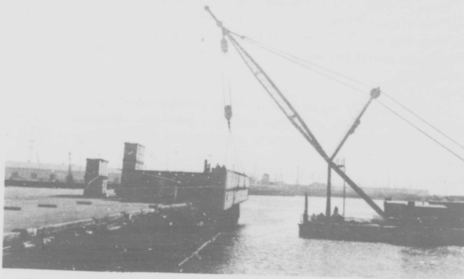
Figure 18. 2 x 30 causeway about to be launched from vertical position (11-ft rail height).
