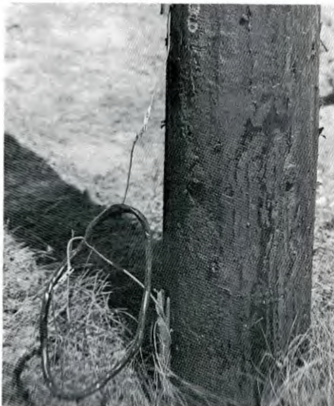
Figure 12. Wire loop inserted in ground lead for impedance correction.
