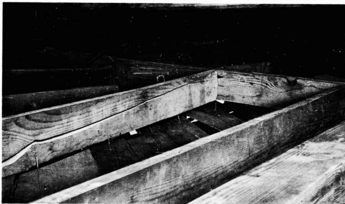
FIGURE 37. Barracks damage, Test 1.
