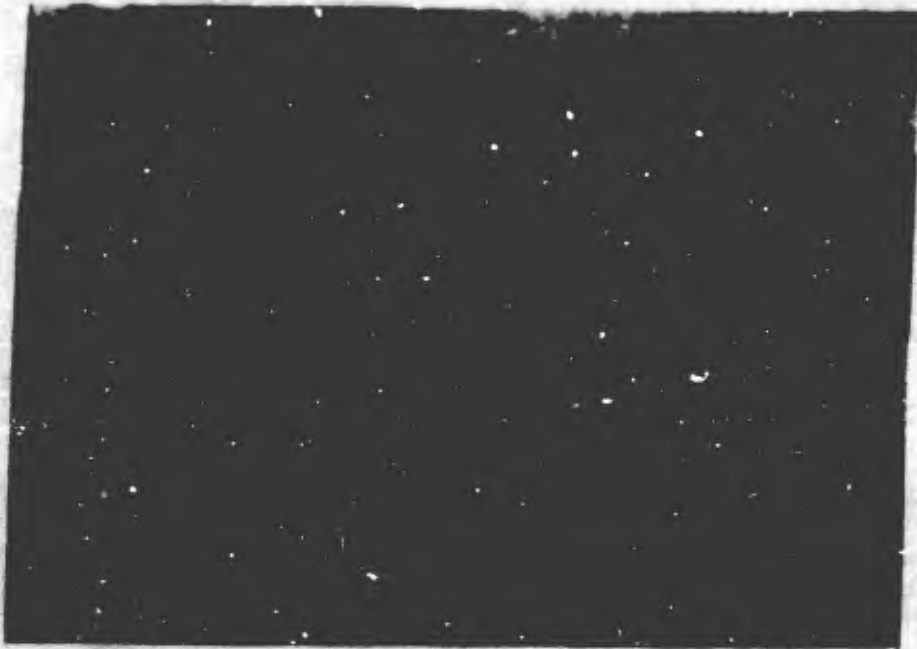
Figure 139. Crack and settling in the concrete floor of the Anadyr' fish cannery. The rulers show the amount of settling of the floor of the building. Photo by S. P. Kachurin.
