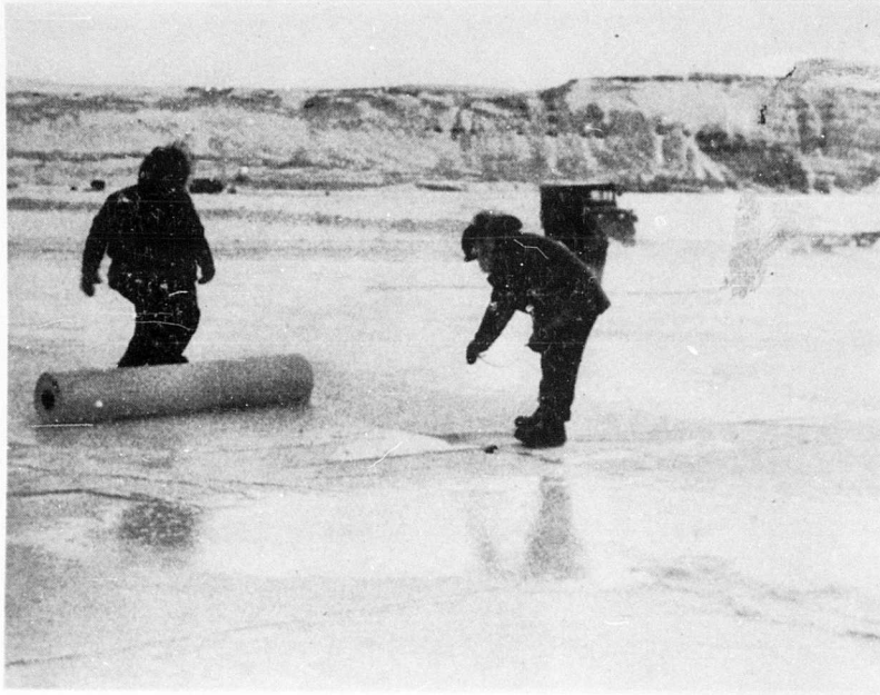
FIG. 4.11. Laying Fiberglas reinforcement in flood water on Parking Apron No. 2 (official photograph, U.S. Navy)
