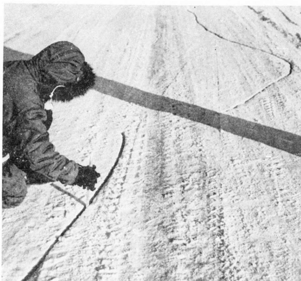
FIG. 8.1 Runway crack at North Star Bay runway
