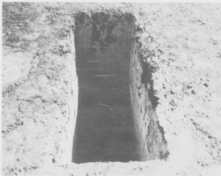
Fig. 8. Unit 25A. Top: pre-shot, ground zero toward right lower corner; bottom: post-shot, ground zero to left (note cracks around side walls and bow in walls).
