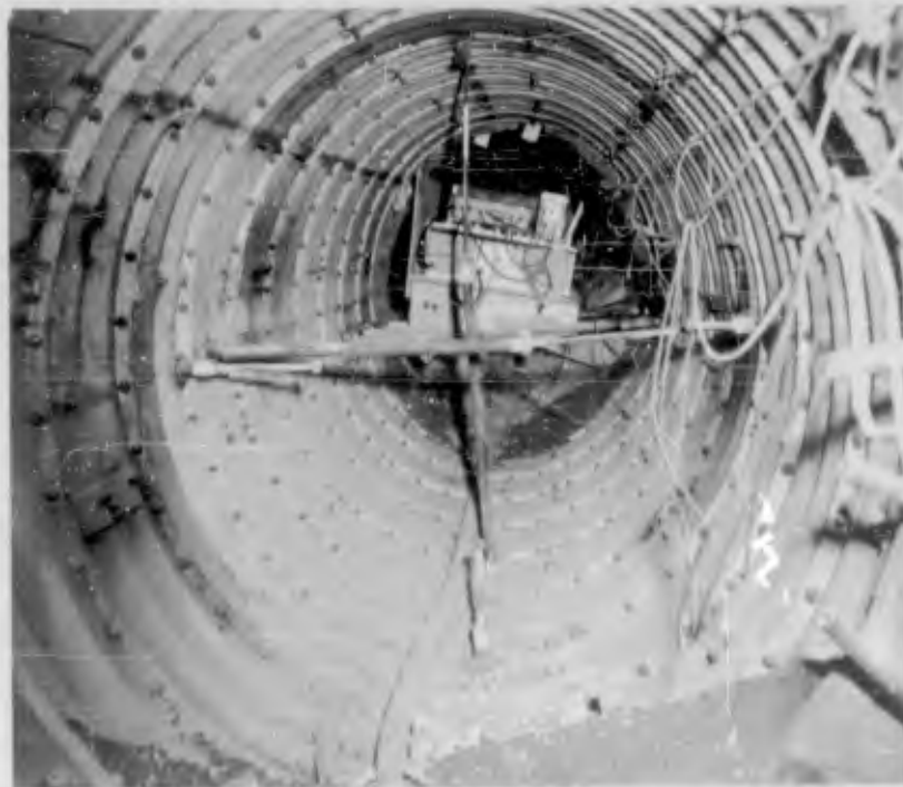
Figure 3.50 Test Section C6c (postshot) (DASA - NOU 228-03 NTS-62).
