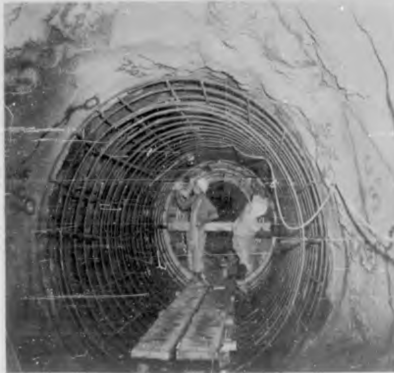
Figure 2.20 Reinforcing steel installed, ready for concrete form; concrete liner cast against rock. (LRL Photo, 1960).
