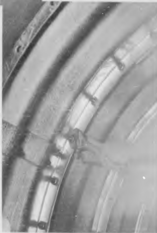
Figure 2.5 Tightening of bolts connecting one ring of corrugated steel tunnel liner to the next ring. (H&N-AEC 796-5, 1960).
