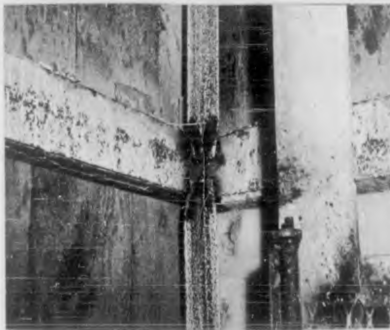
Figure 3.6 Shaft Sta 1+35, SW corner of bearing set. Note failure of hanger angles. (H&N-AEC 62-1241-5, 1962).
