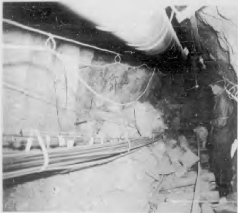
Figure 3.11 Access tunnel from Sta 2+10, approximately 595 feet from zero point, looking north (post-shot) (DASA - NOU 160-02 NTS-62).
