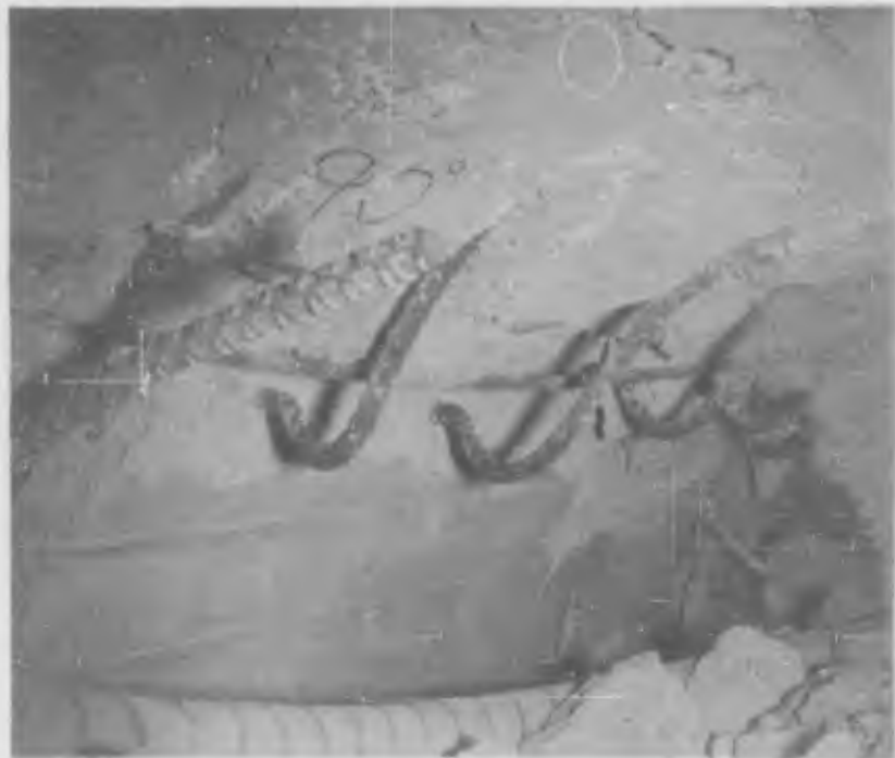
Figure 3.87 Close-up view B3d (postshot). Note buckled reinforcing bars at 90° (DASA - NOU 324-03 NTS-62).
