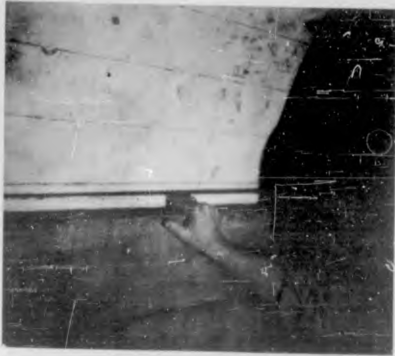
Figure 2.32 Installing wood lagging between wide-flange rings and foam units (DASA - NOU 037-12 NTS-62).
