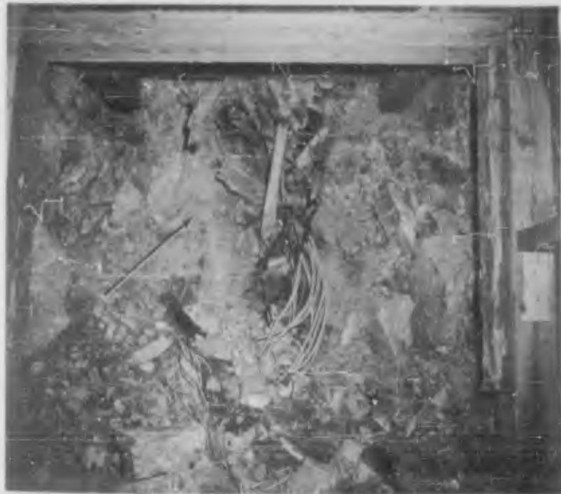
Figure 3.21 Access tunnel from Sta 4+85, approximately 325 feet from zero point, view to north (post-shot). Note crushed timber sets (DASA - NOU 365-05 NTS-62).
