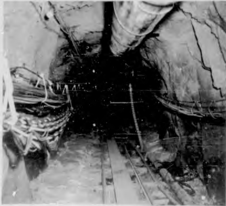
Figure 3.10 Access tunnel from Sta 2+00, approximately 605 feet from zero point, looking north (pre-shot) (DASA - NOU 085-11 NTS-62).
