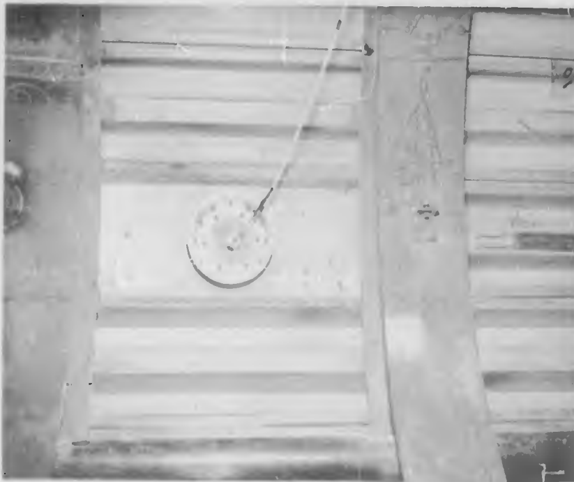
Figure 2.41 Pressure gage installed in corrugated steel liner (DASA - NOU 072-04 NTS-62).
