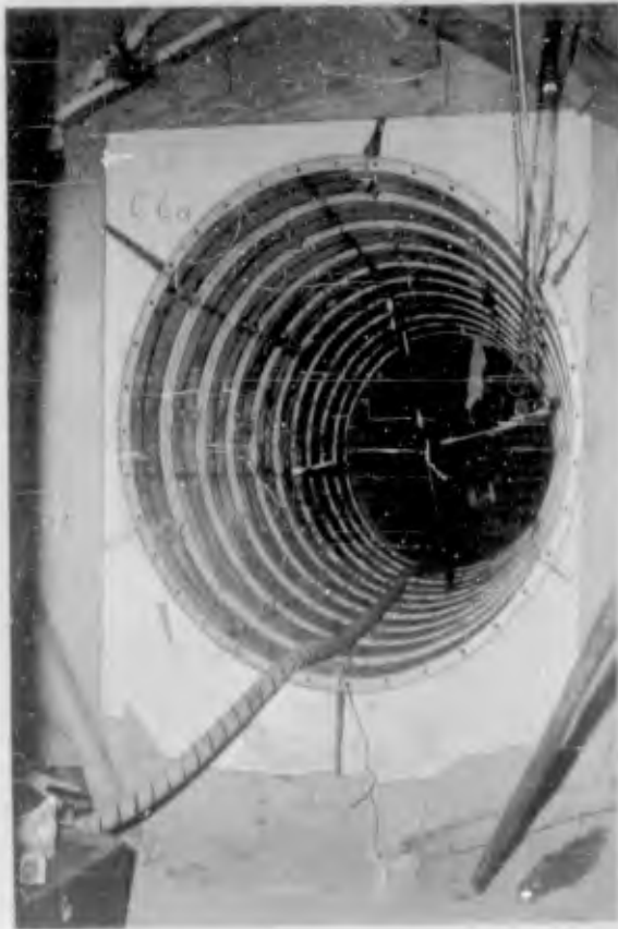
Figure 2.36 Completed liner composed of tunnel liner plates and precast foam (DASA - NOU 082-02 NTS-62).
