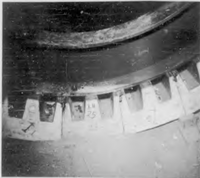
Figure 2.27 Panels installed at invert. Note sand bed and wood blocks holding panels against wide-flange rings (DASA - NOU 044-08 NTS-62).
