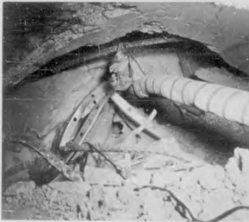
Figure 3.84 East end of B6a as viewed from B3d (postshot). Note collapsed tunnel liner plates (DASA - NOU 324-05 NTS-62).
