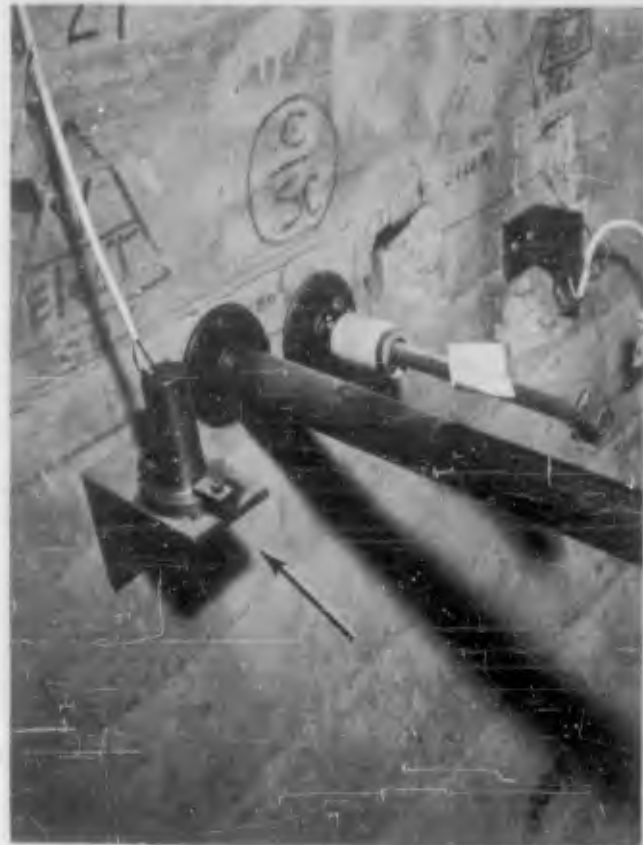
Figure 2.44 Velocity gage installed on reinforced concrete liner (DASA - NOU 082-02 NTS-62).
