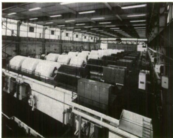
FIG. 3. Compressor/exhauster sets in the Air House.
