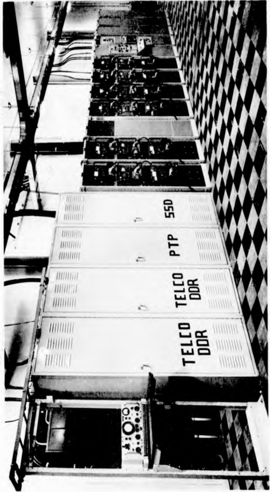
Fig. 1-7 Equipment line, west side of equipment room
