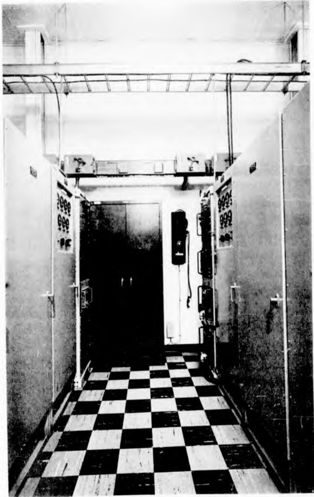
Fig. 1-10 Frequency division data link installation (east side, equipment room)
