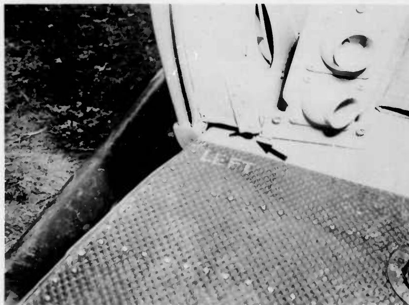
Figure 14. View of left vertical support at floor showing failure and impending separation at attaching point.
