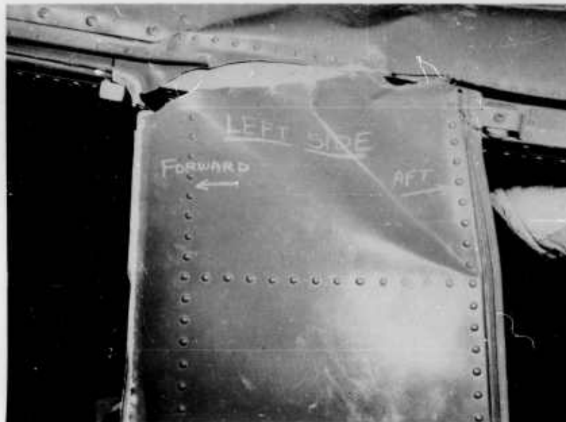
Figure 9. Side view showing failure of left vertical support at upper attachment and shifting of overhead cabin structure.
