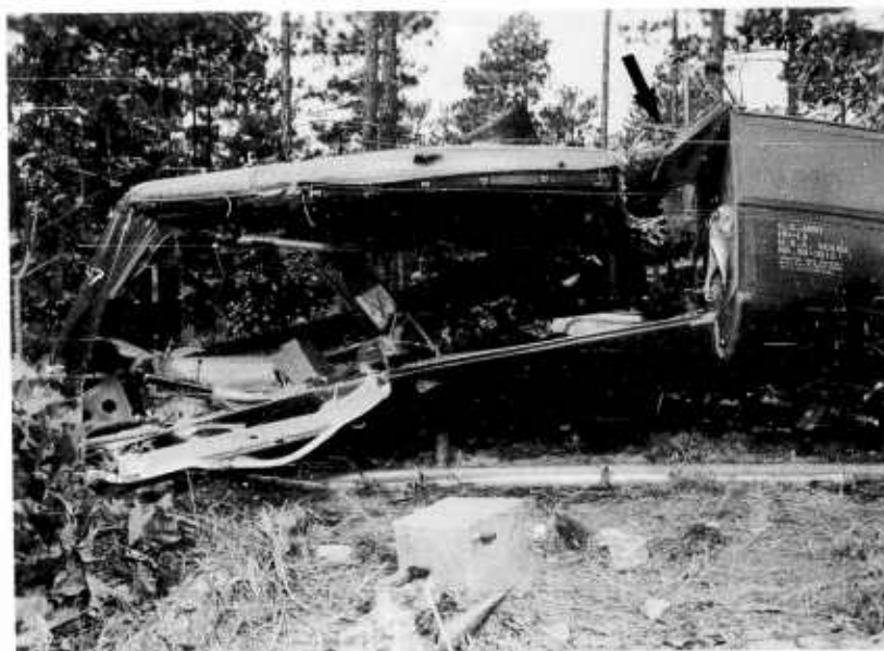
Figure 23. Wiring was the remaining support of the roof structure in Accident "D".
