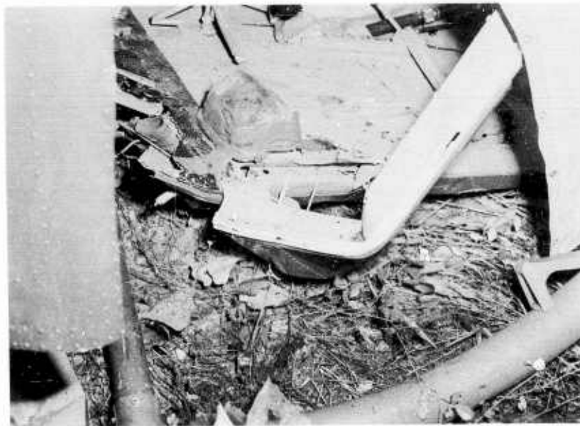
Figure 16. Wiring supported the bottom on the right side support in Accident "D".
