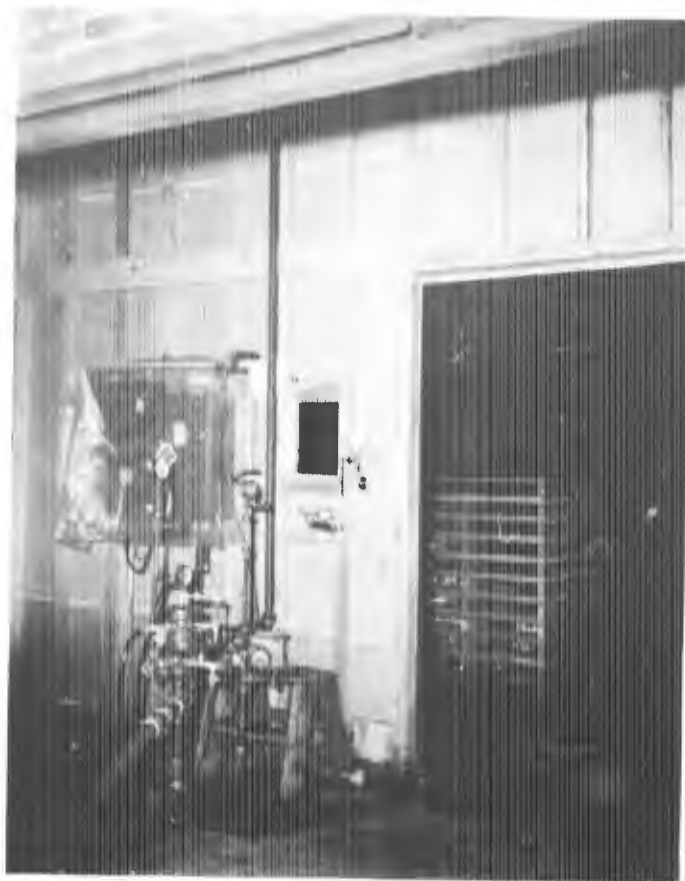
Water System Test Set-up
