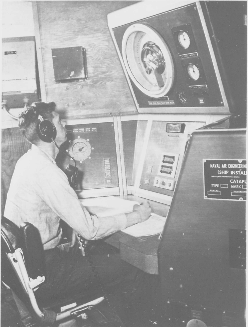
Figure 6 - CVA67 Wrap-Around Control Console (NAEL(SI) PN 612619-1) Installed in TC13 Mod 1 Control Room
