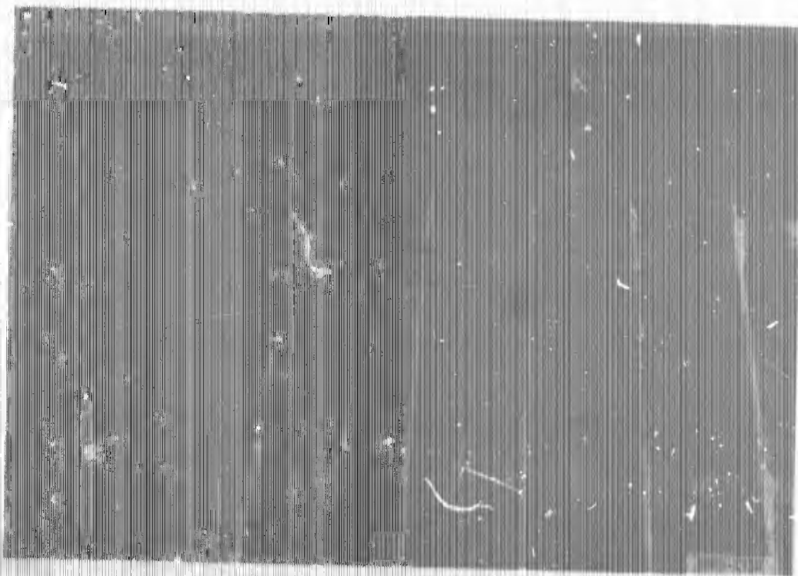
Photograph 3. Typical overlapping edge breaks adjacent to an end joint
