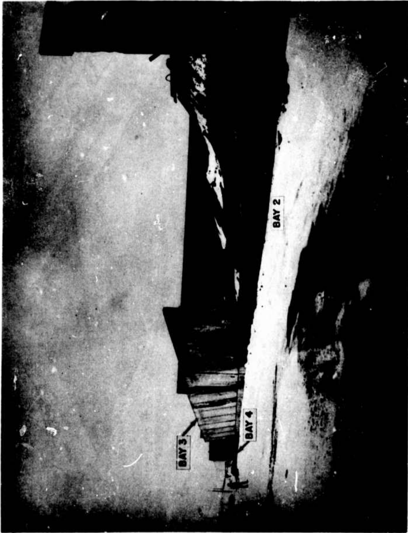
Figure 254. Elmendorf AFB Warehouse (Failed reinforced-concrete roofbeam seat--small horizontal ties were insufficient to resist lateral load)
