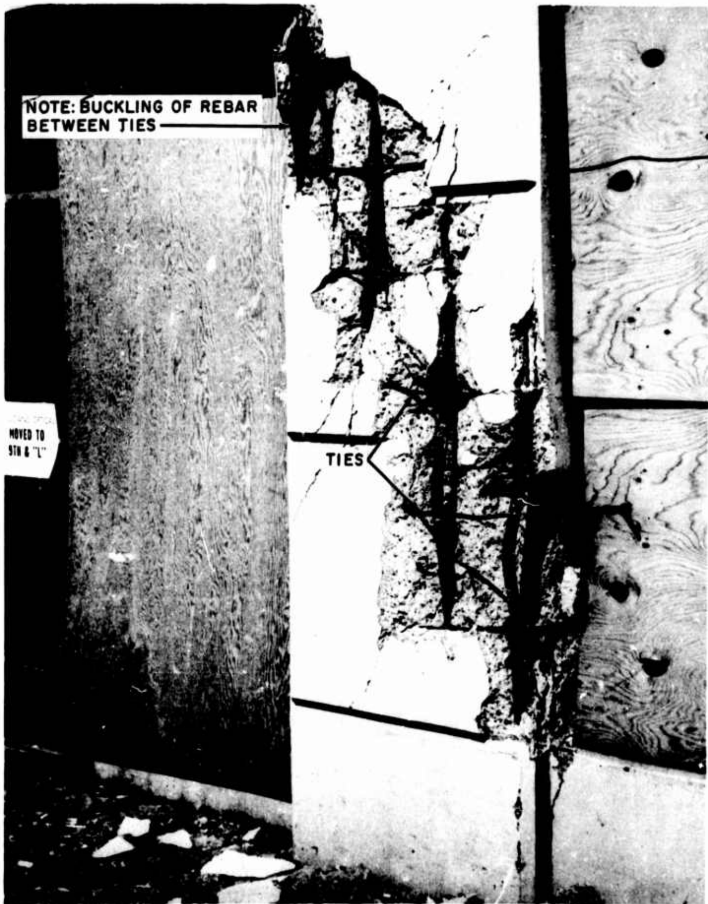
Figure 155. Mount McKinley Building (Shortened column in south wall near southeast corner of structure)
