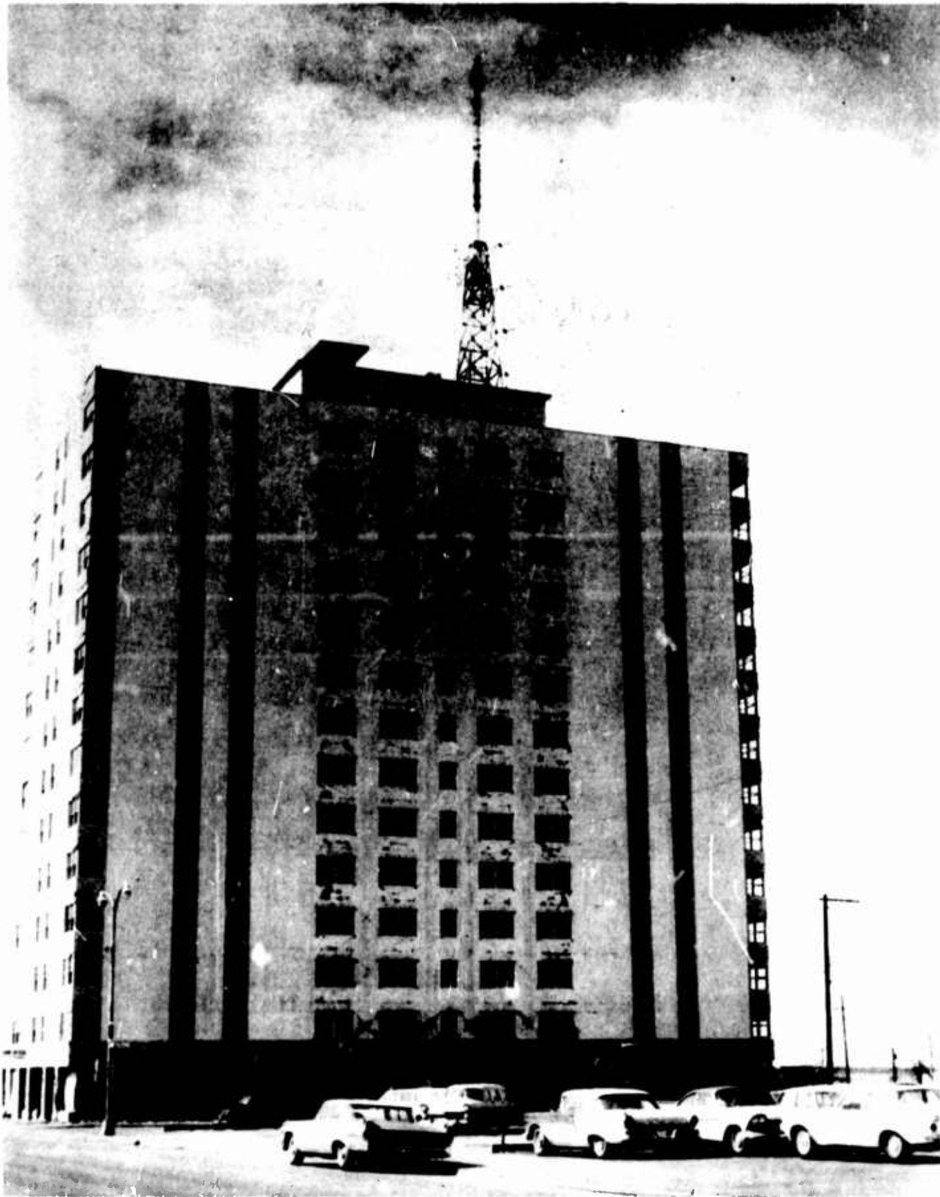
Figure 144. Mount McKinley Building (East side of the fourteen-story reinforced-concrete structure showing diagonal tension cracks in spandrel walls)
