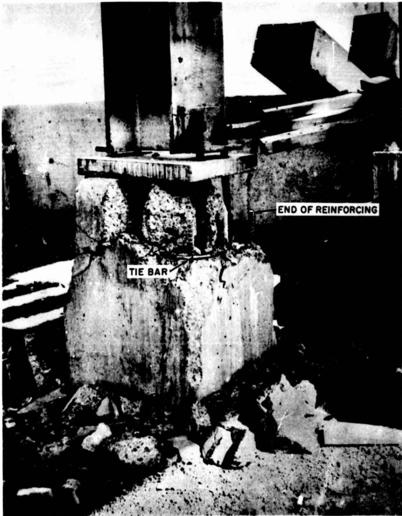
Figure 225. Alaska Brewery Company Structure (Damage to an interior footing, mainly above first horizontal tie)
