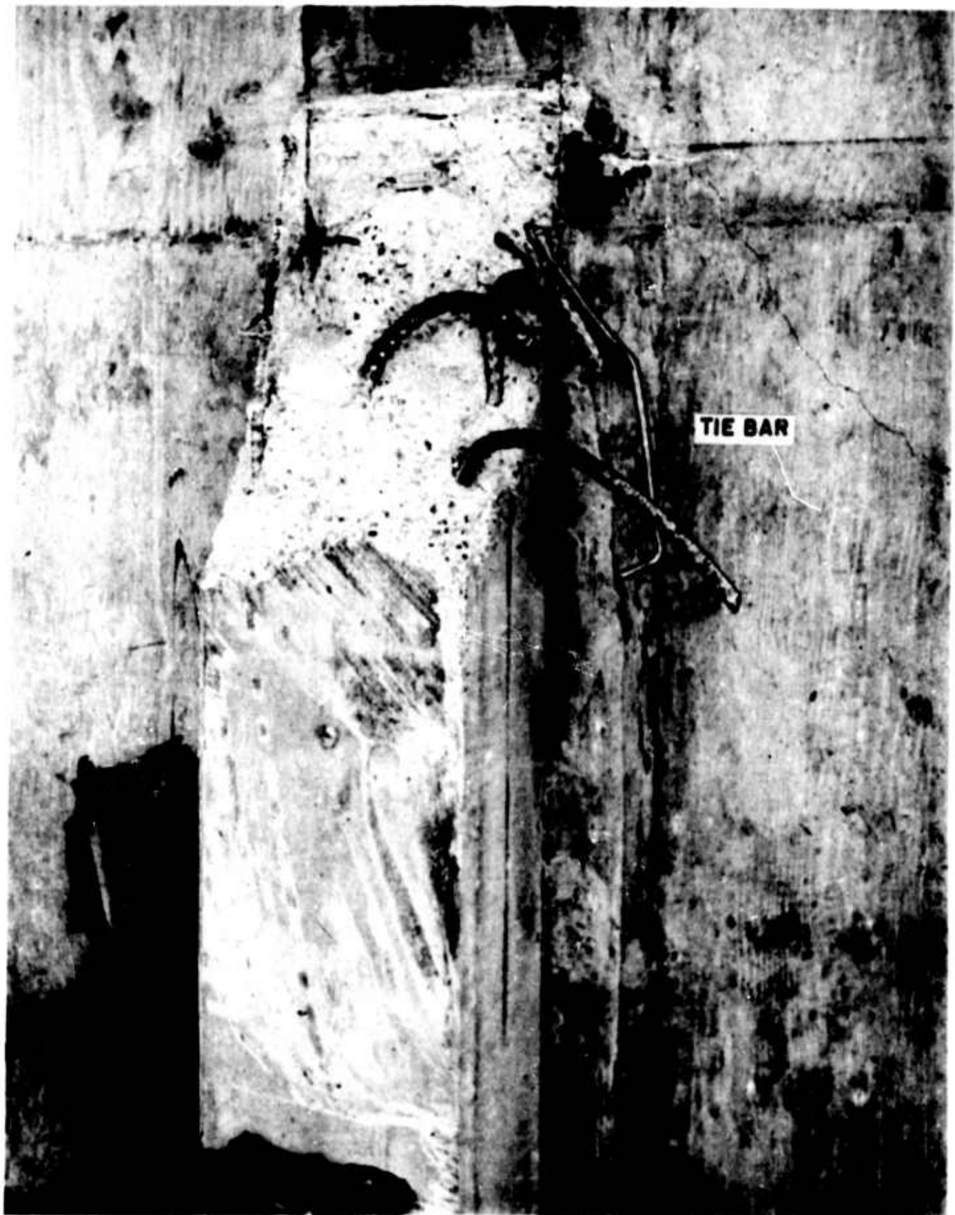
Figure 261. Elmendorf AFB Warehouse (Closeup of column failure showing tie-rod failure)
