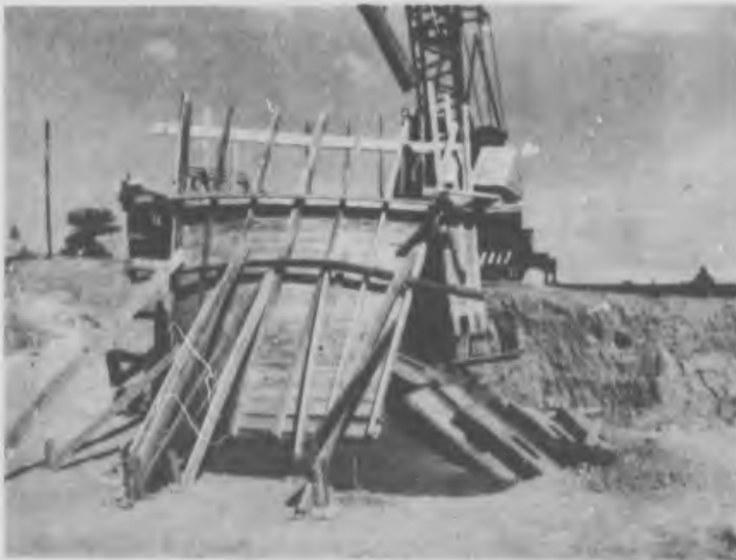
Fig. 30. Collapse of wall with lead weights crashing down. F8074
