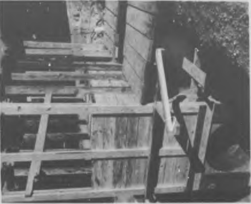
F807C Fig. 17. Initial height of sandbox extended to 8 feet; height of fill over crown of liner is 5 feet.
