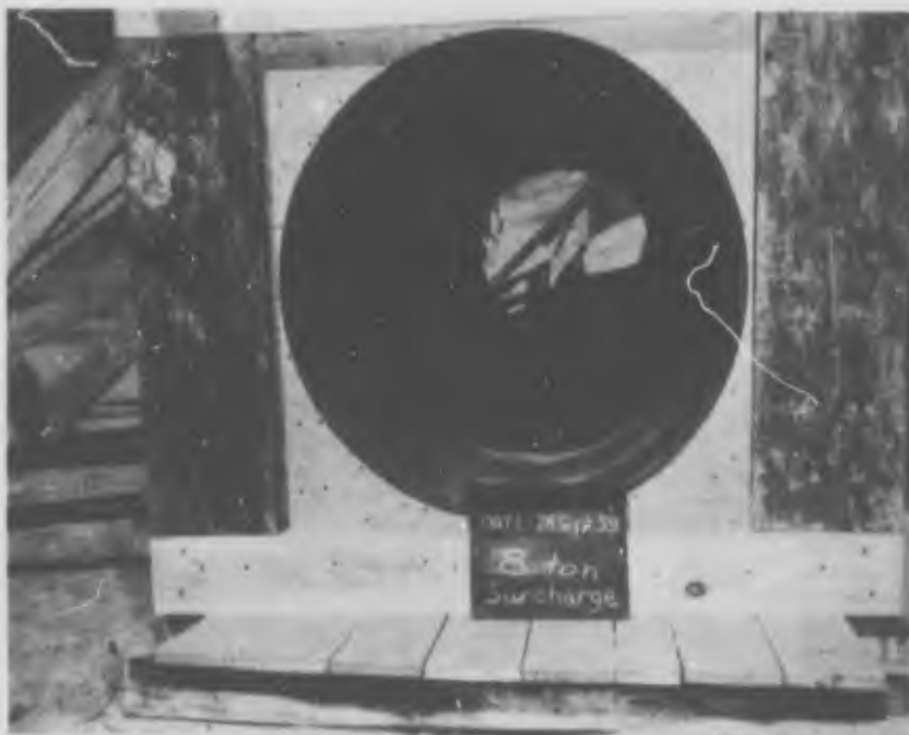
Fig. 22. Ring deflections from south end of liner at 8-ton level (Ring No. 1 in foreground).
