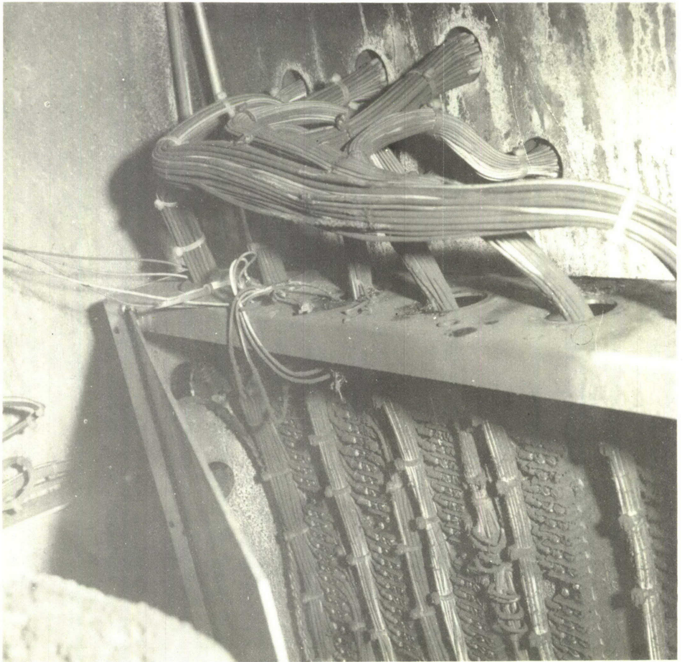
Figure 13 Interior of Junction Box
