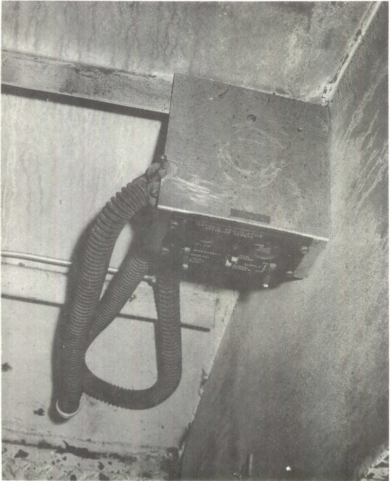
Figure 8 Test Cell Oxygen Regulator
