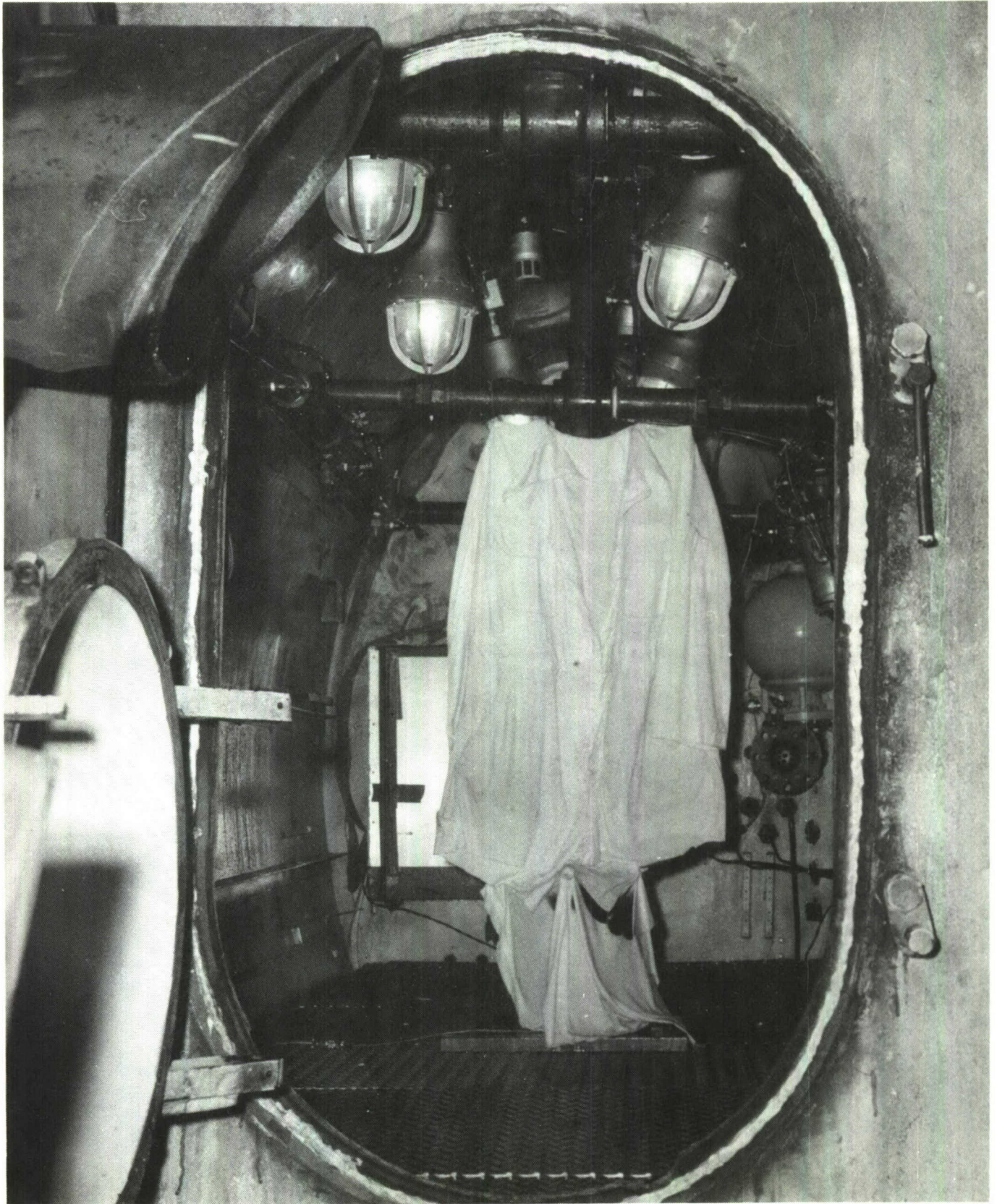
Fig. 6 Typical Conditions After Water Spray Fire Test
