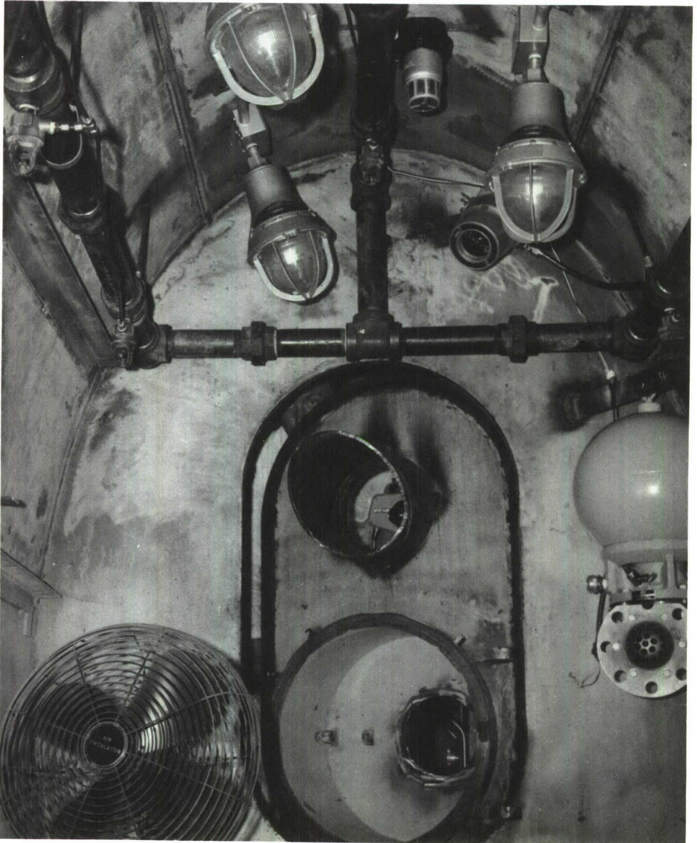
Fig. 3 Inside Test Chamber - West End at Door to Interlock Section 74
