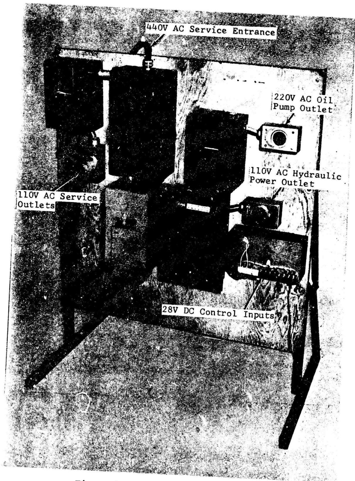
Figure 39. Power Distribution Panel.
