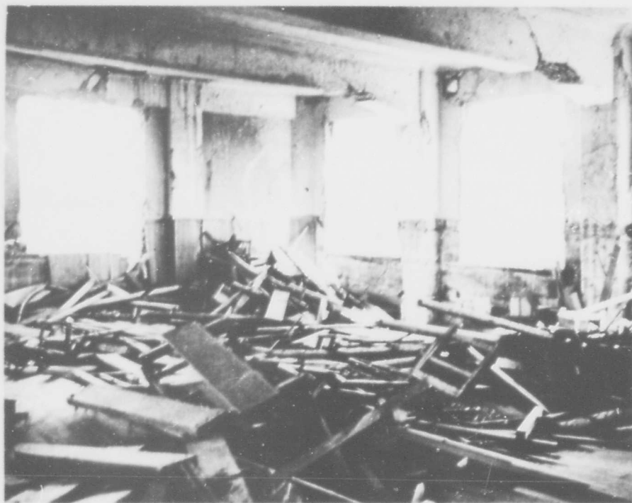
Figure 19. Nagasaki elementary school second floor corner facing blast about one-fourth mile from zero. Undisturbed contents in September 1945. It is suggested that cylindrical vortices formed on the four edges of each window aperture and crept along the walls and ceiling tearing off the wainscot and sound-proofing panels by their violent action. The debris was left in rough circular distribution on the floor probably by waves reflected from the walls and corner (see Figures 14 to 18). The large lumber was from benches and tables. The school was not occupied at the time. Lethal casualties would result from missiles, blast, and ionizing radiation at this location.
