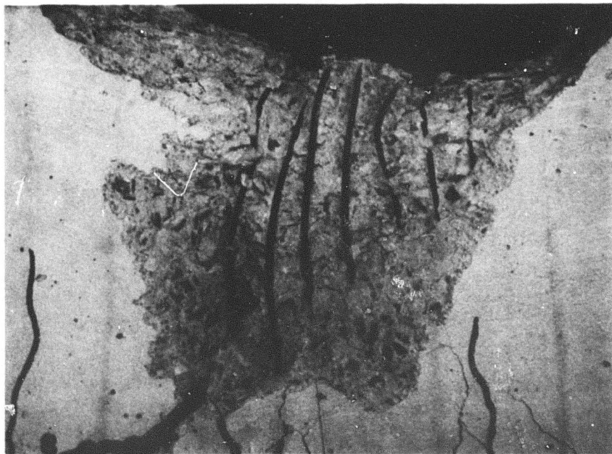
Photograph 17. Beam F-2 at failure
