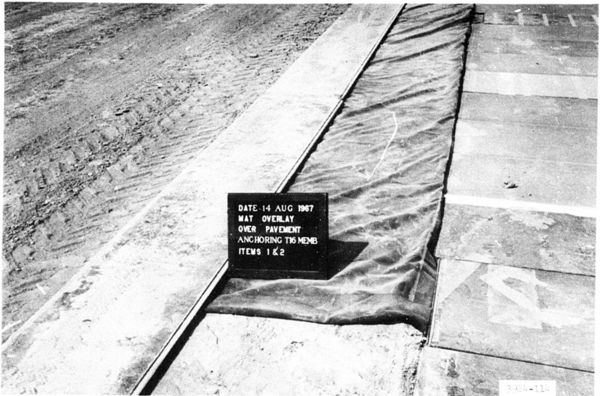
Photograph 35. Free edge of T16 membrane anchored with landing mat
