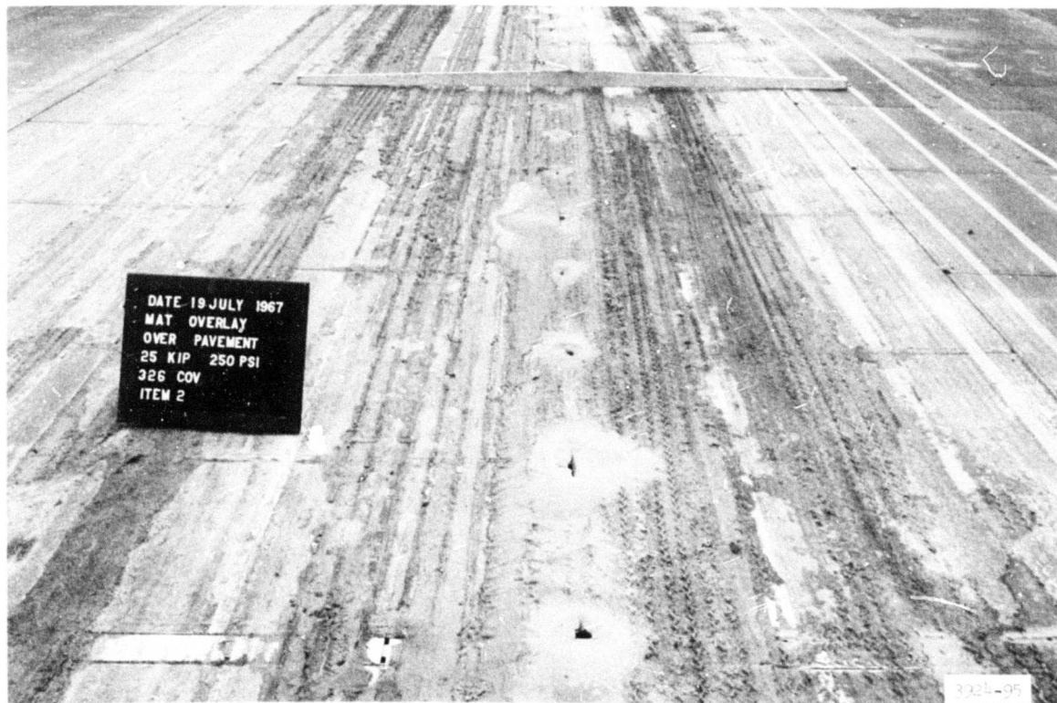
Photograph 24. Item 2 after 26 coverages applied during heavy rainfall caused severe pumping (326 coverages total)
