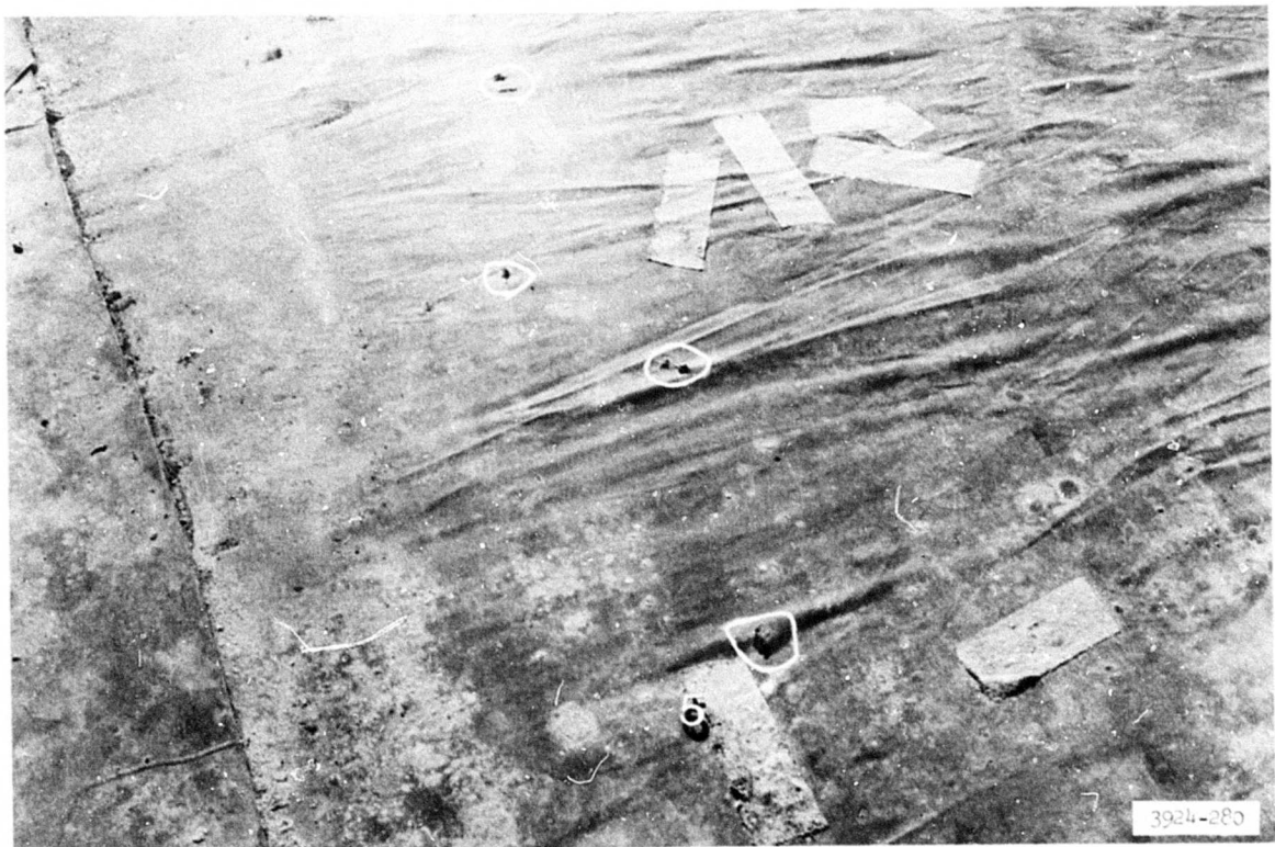
Photograph 63. Small holes cut in T16 membrane in item 5
