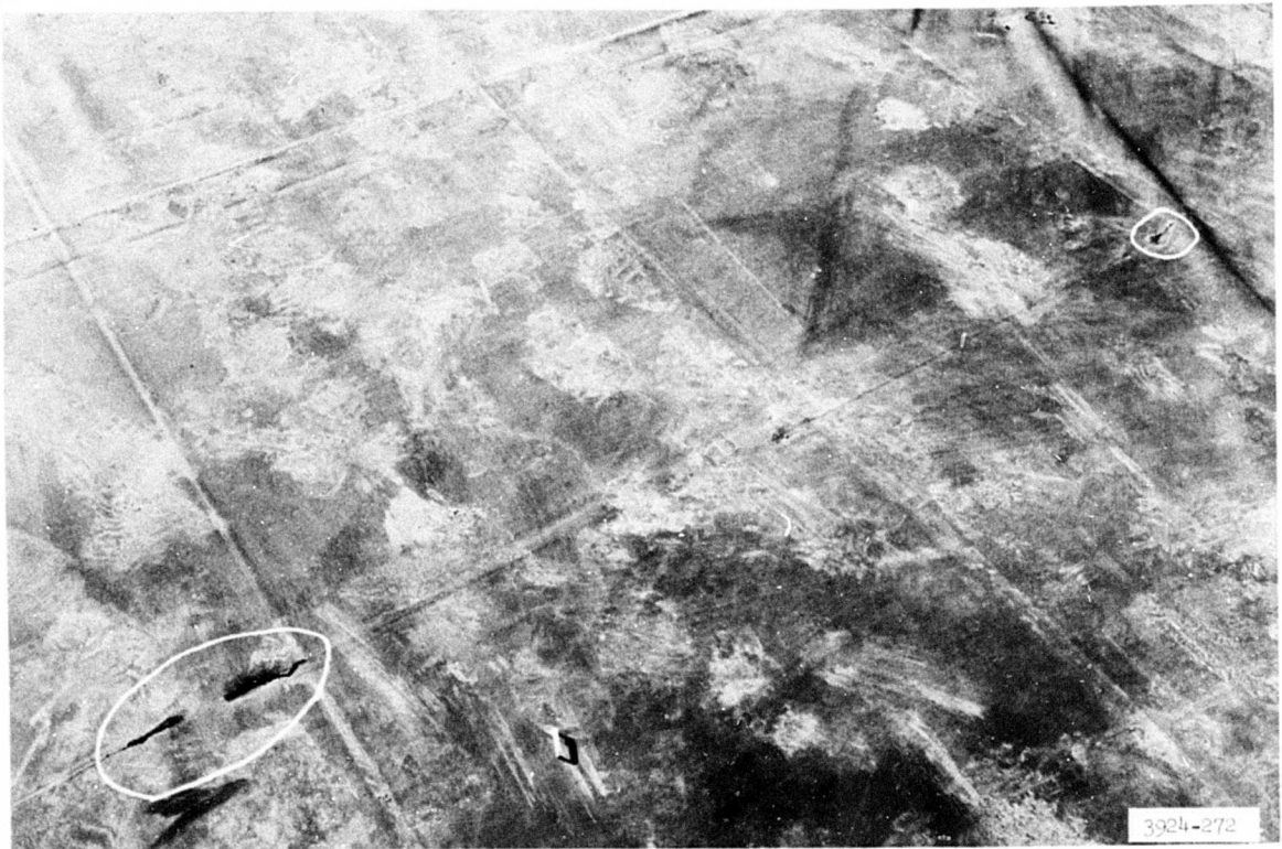
Photograph 57. Membrane cut by pinching action of mat in item 1
