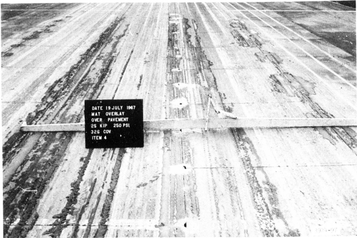
Photograph 26. Item 4 after 26 coverages applied during heavy rainfall caused severe pumping (326 coverages total)
