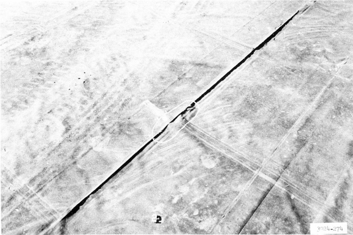
Photograph 58. Membrane cut by pinching action of mat in item 2
