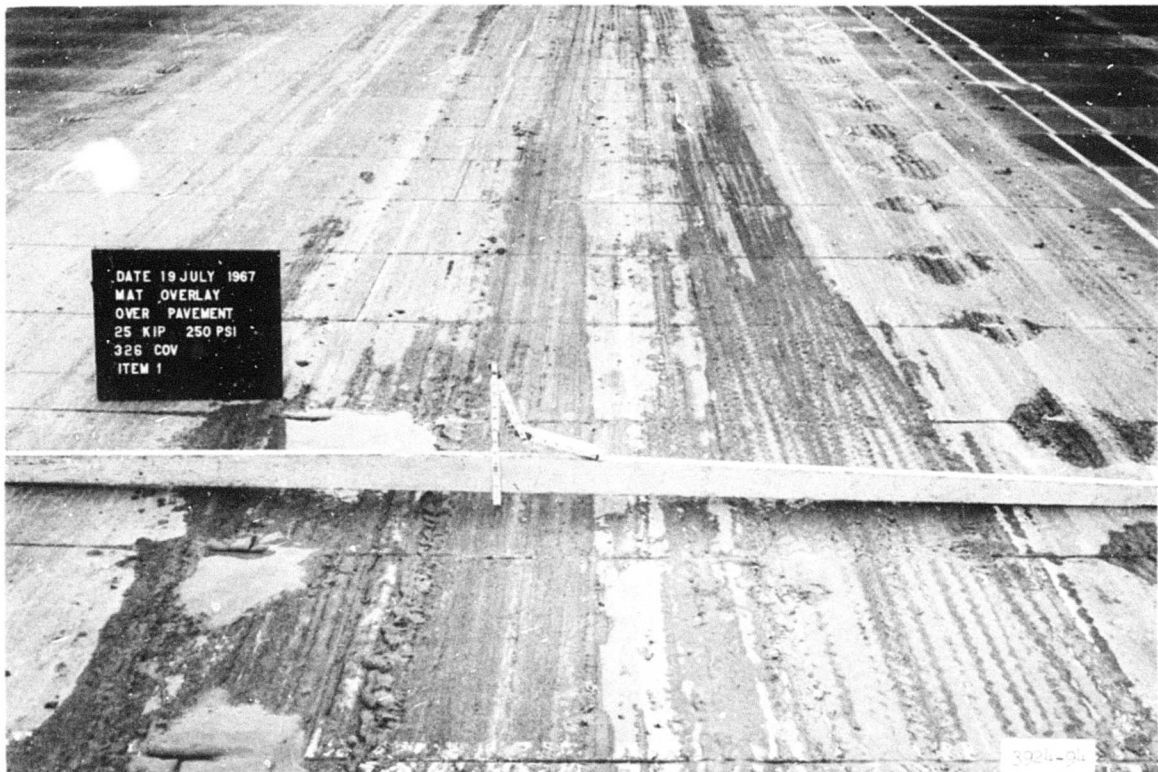
Photograph 23. Item 1 after 26 coverages applied during heavy rainfall caused severe pumping (326 coverages total)
