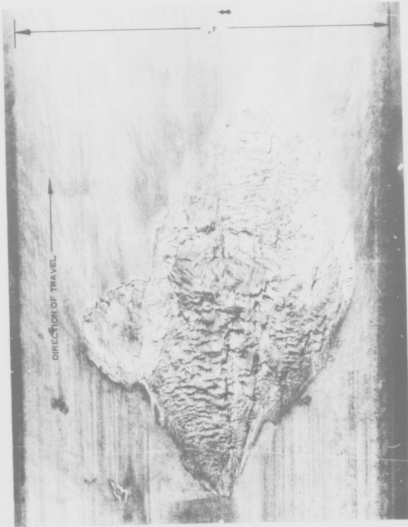
FIGURE 14 GOUGE ON TOP SURFACE OF RAIL
