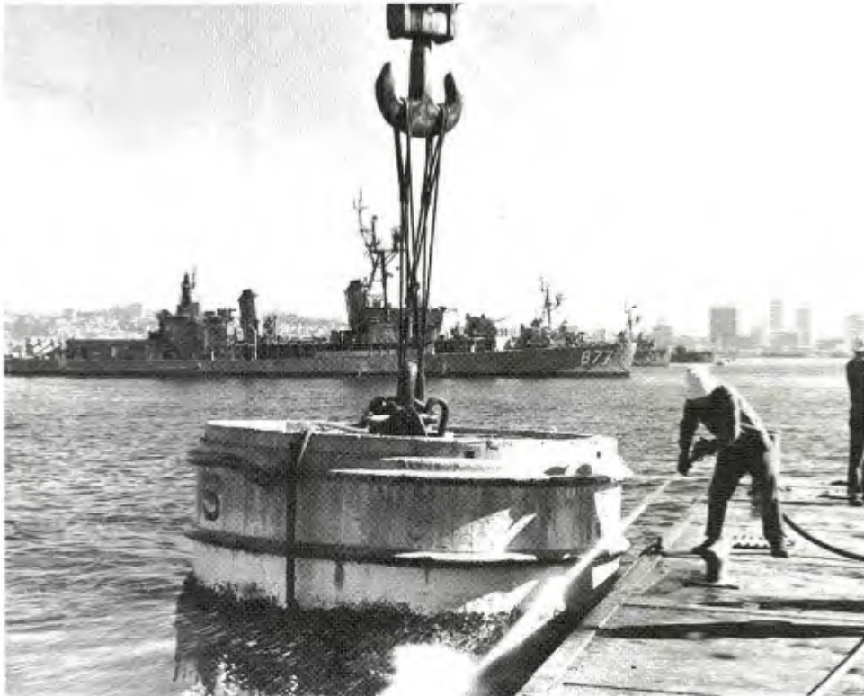
Figure 1. Hosing of marine fouling from hand lay-up buoy in San Diego Bay.
