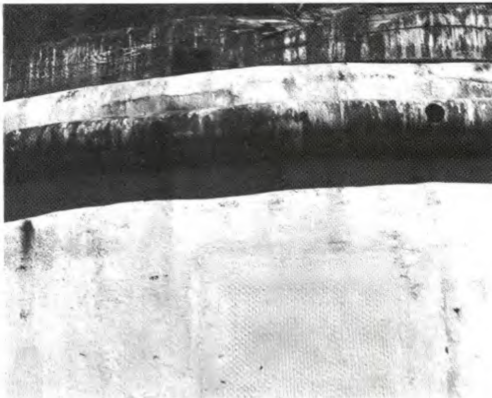
Figure 4. Upper portion of spray-up buoy in San Diego Bay after 4 years of service. Note worn upper wooden fender, deteriorated shoulder, and square at bottom center.
