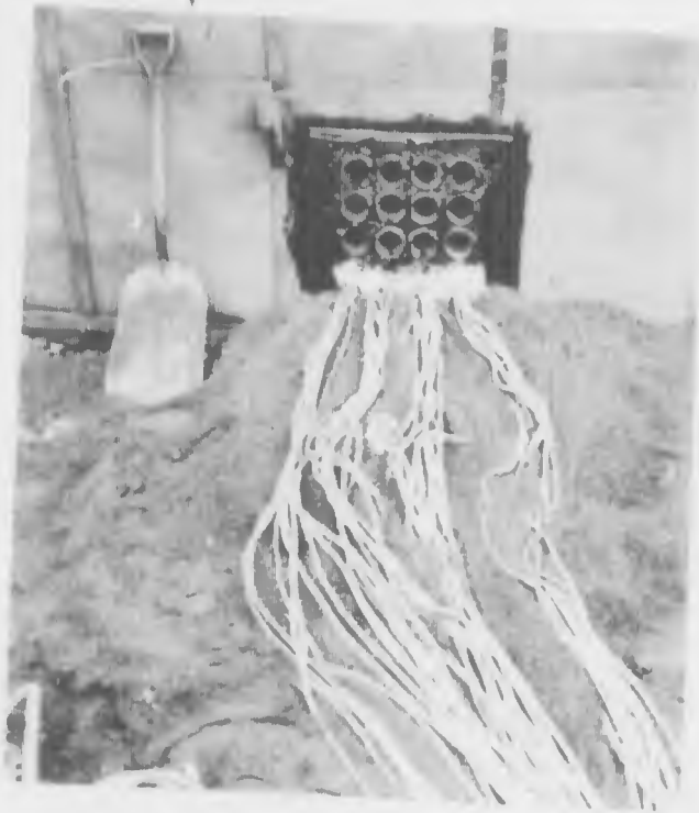
Figure 1. Entrance of thermocouple leads to instrument room
