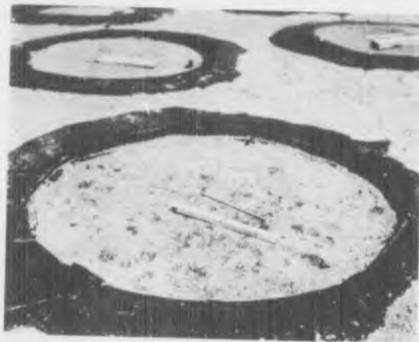
Figure 2. Settlement of pavement in Element W on 11 April 1947
