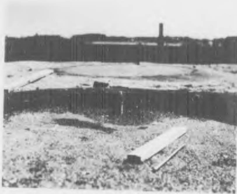
Figure 1. Settlement of pavement in Element H on 11 April 1947
