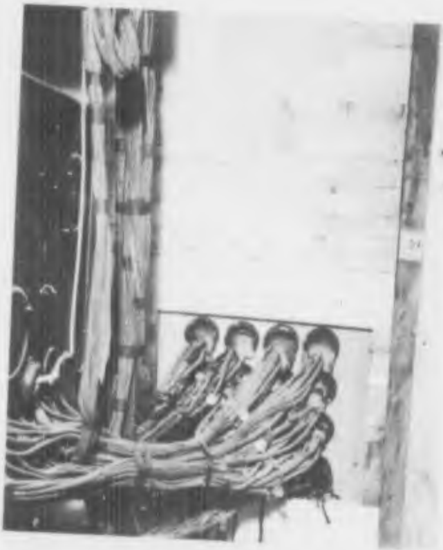
Figure 2. Thermocouple leads to instrument DCW FIELD TEST SECTION THERMOCOUPLE LEADS TO INSTRUMENT ROOM
