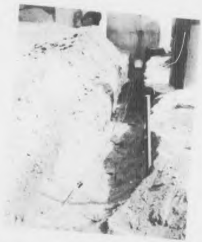
Figure 2. Thermocouple leads in trench from elements to instrument room
