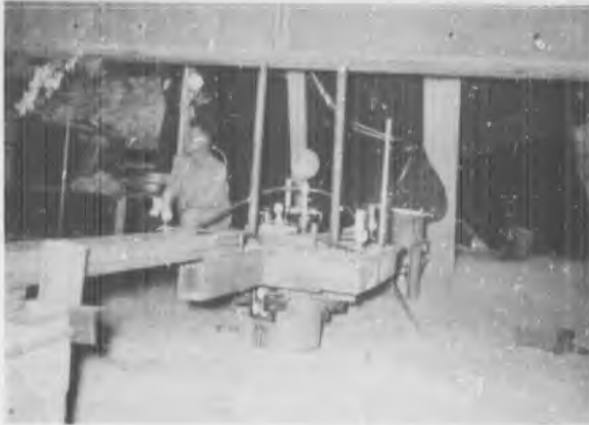
Photo 6-a - Typical Tension Test Loading Apparatus and Instrumentation, Test Pile 16 - 16-In. Steel Pipe Pile
