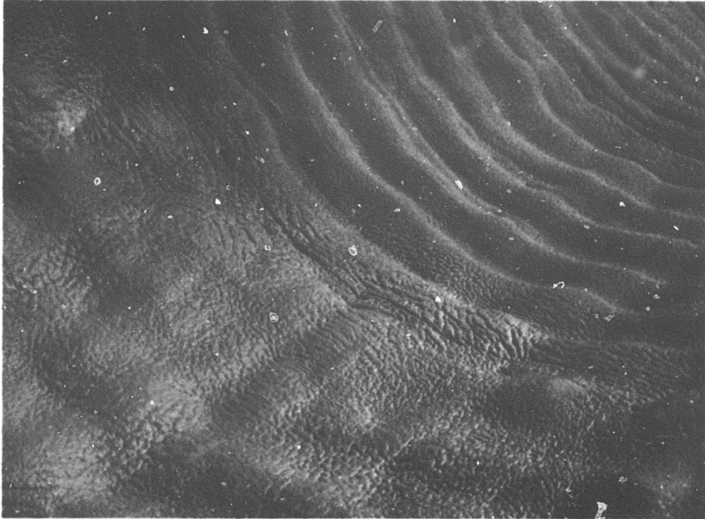
Figure 7. Urethane insulation on interior of corrugated arch. Upper right sprayed parallel to corrugations, foreground sprayed across corrugation.
