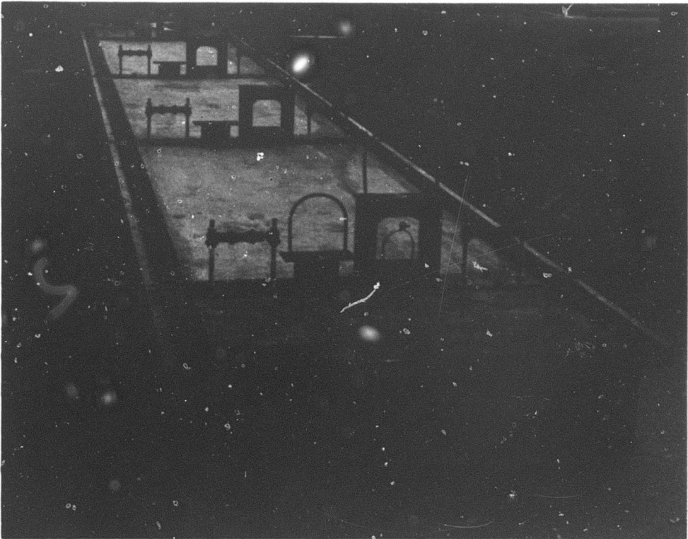
Figure 3. Experimental utilidor with insulated floor panels and pipe supports in place.
