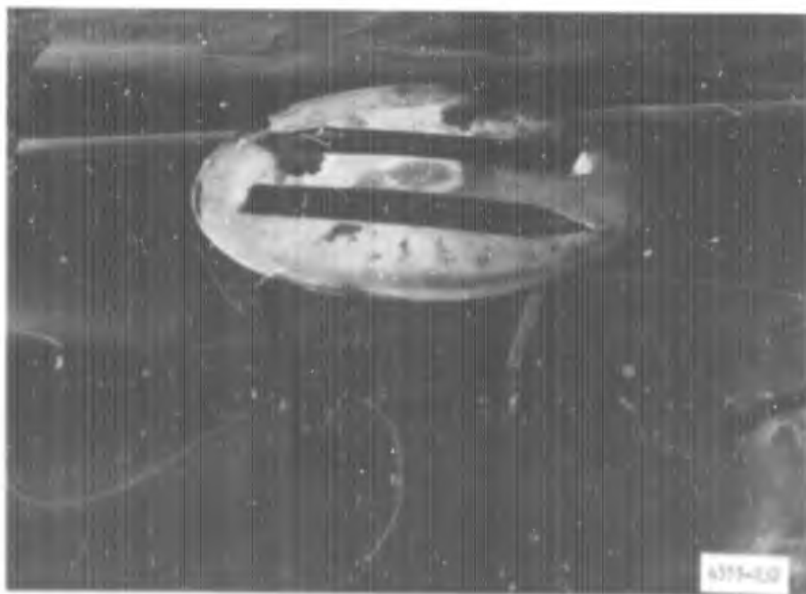
Photograph 6. Two-legged anchor driven through membrane surfacing into the soil subgrade to a depth of 1 in.
