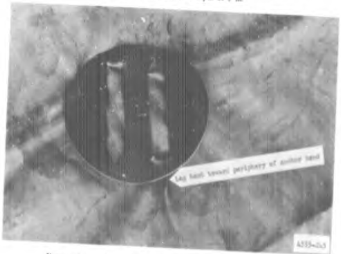
Photograph 12. Anchor with straightened legs driven through membrane into the soil subgrade to a depth of 9 in.
