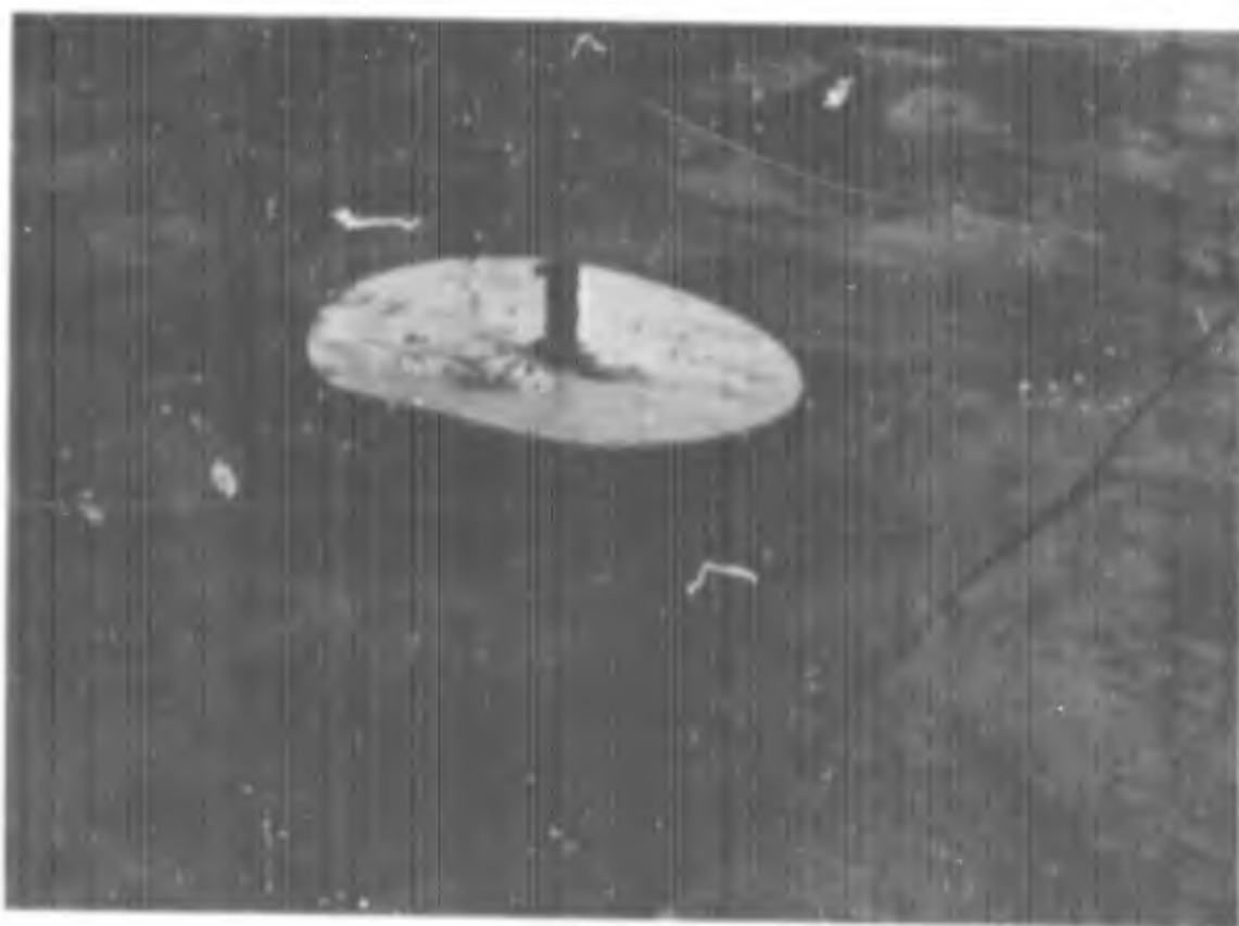
Photograph 2. Head of guy anchor broken from reinforcing bar
