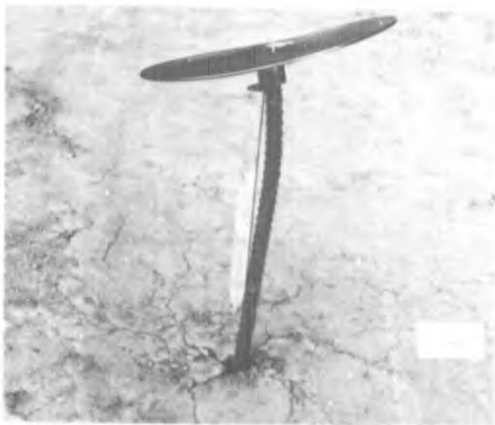
Photograph 13. Threaded guy anchor driven into the soil subgrade to a depth of 6 in.
