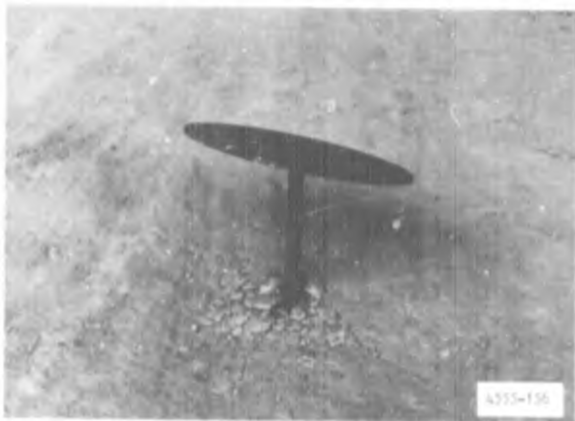
Photograph 16. Guy anchor driven into the soil subgrade to a depth of 18 in.
