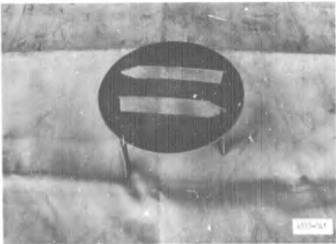
Photograph 10. Legs of two-legged anchor straightened to a vertical position and driven through membrane into the soil subgrade to a depth of 2 in.
