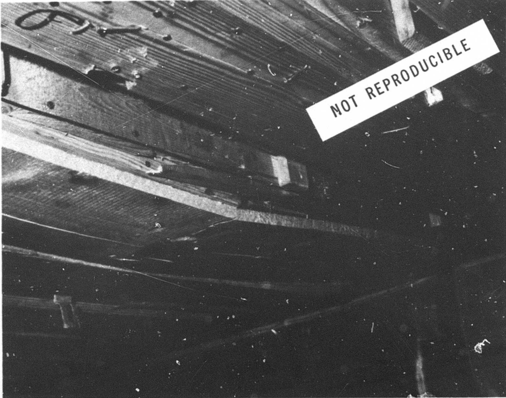
Figure F-10. Damage to roof beams from two 81-mm rounds.
