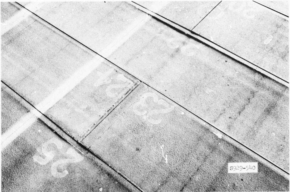
Photograph 7. Splits and depressions in the top skins of panels 22 and 25 after 340 coverages
