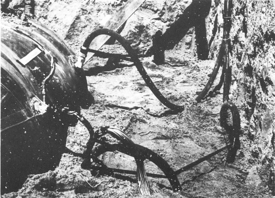
Figure 17. Looping of instrumentation and pressure lines to prevent damage from ground motion.
