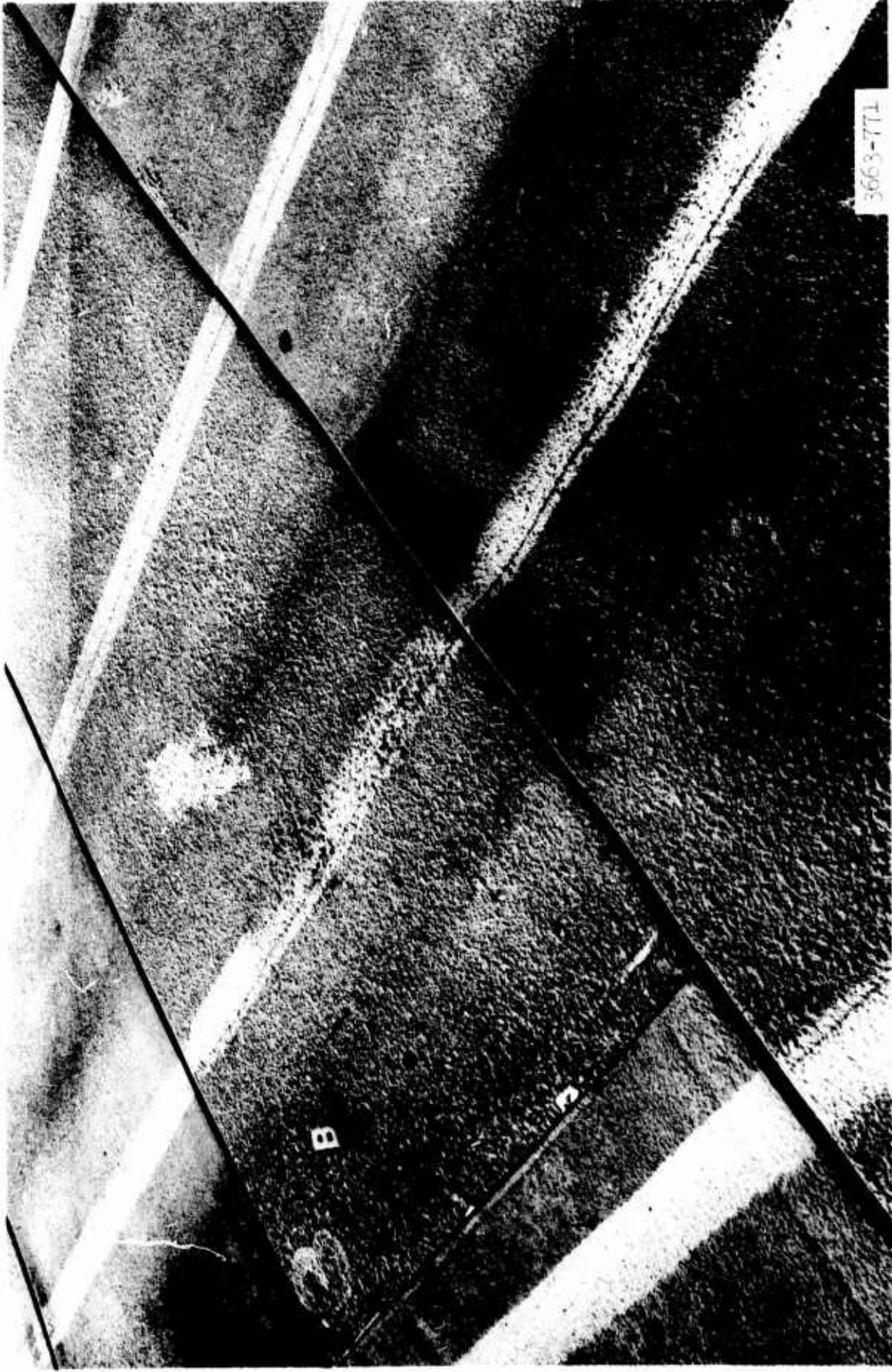
Photograph 11. Dish in mat plank indicating core failure
