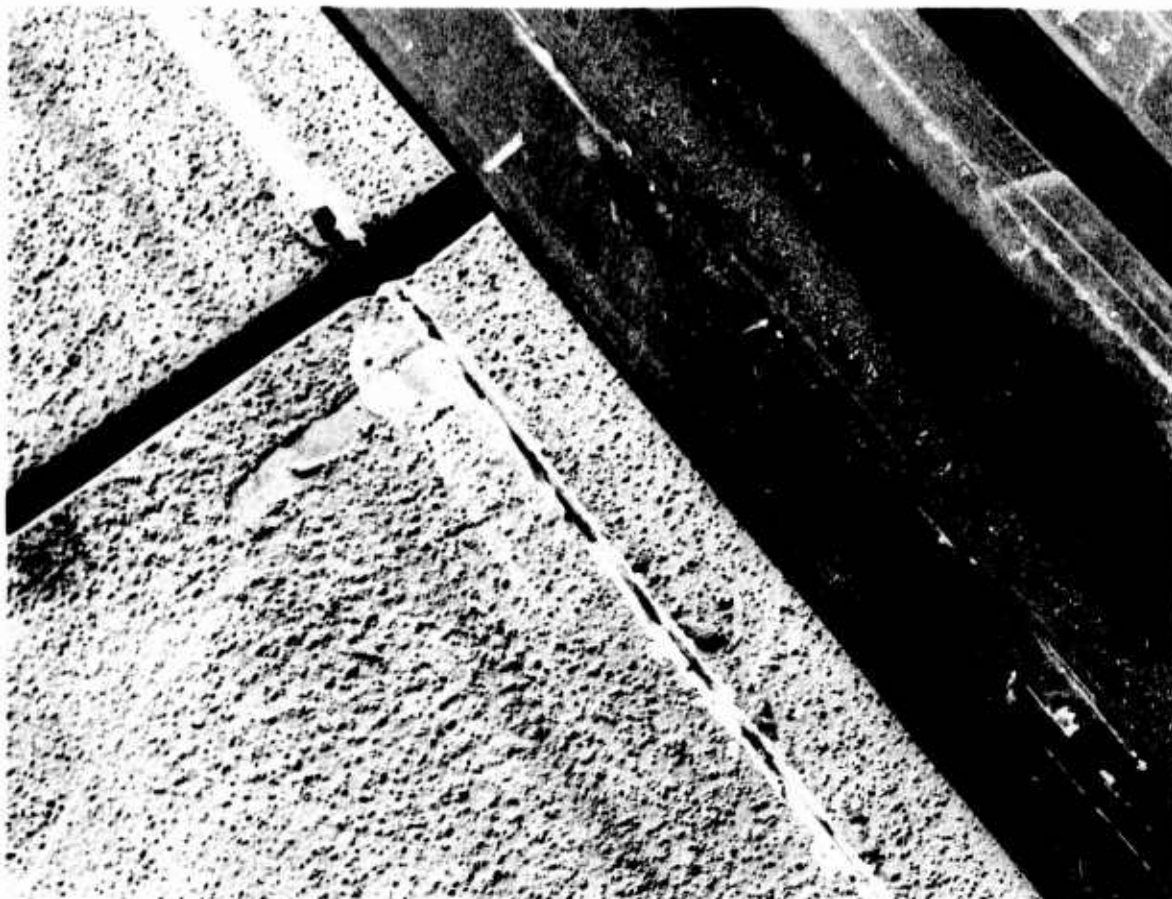
Fig. 7. Close-up of end-joint failure, lane 1, item 4
