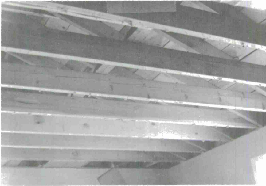
Fig. A-7. Posttest Ceiling Damage, Upstairs Rear North Bedroom
