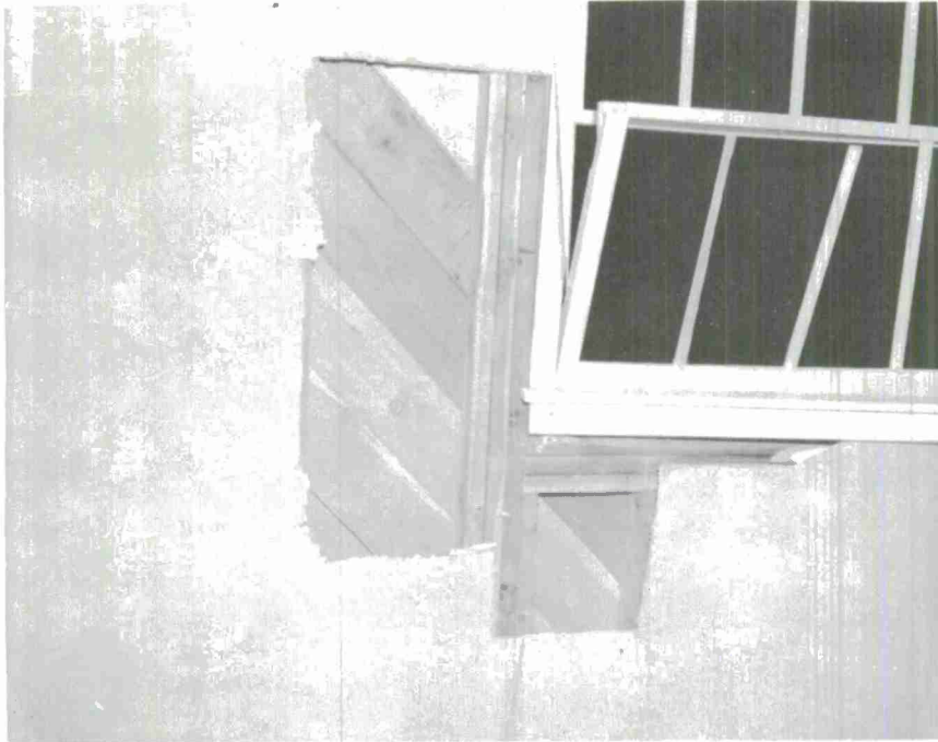
Fig. A-9. Posttest Upstairs Front Bedroom, North Side
