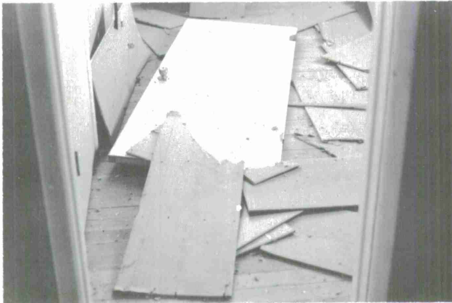
Fig. A-8. Posttest Door and Ceiling Sheathing on Floor of Upstairs Rear North Bedroom
