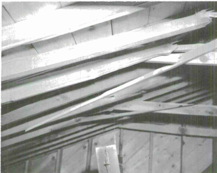
Fig. A-18. Posttest Attic, Westside, View Looking South
