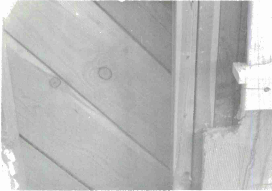
Fig. A-5. Pretest Close-up of Cracked 2 by 4, North Bedroom, Front Window
