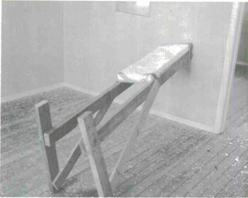
Fig. A-13. Dining Room East Wall, Showing Damaged Glass Trap
