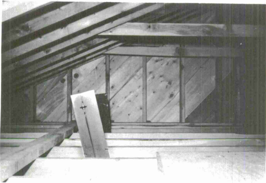
Fig. 3. Maximum Displacement Gage Installed in Attic
