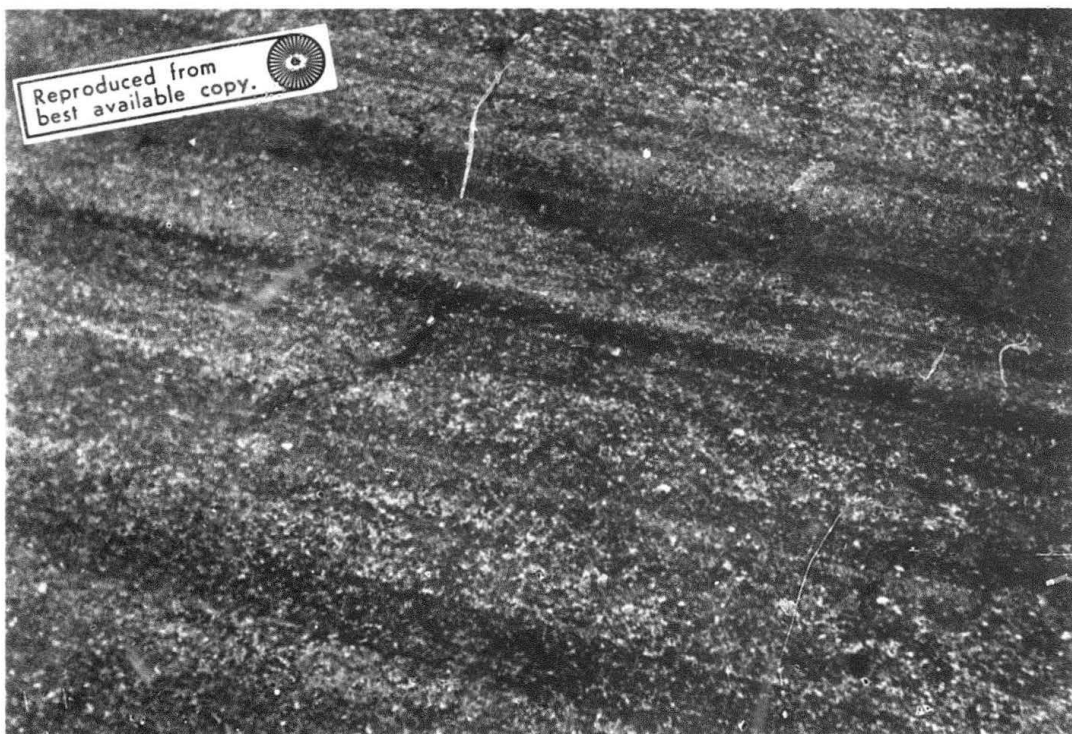
Photograph 3. Distressed area near north end of runway
