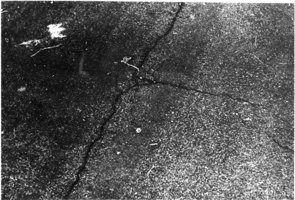
Photograph 4. Typical condition of taxiway pavement
