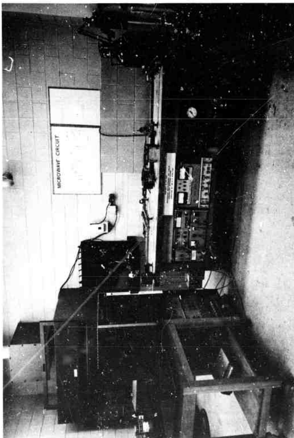
Figure 14. Control Panel and Instrumentation.
