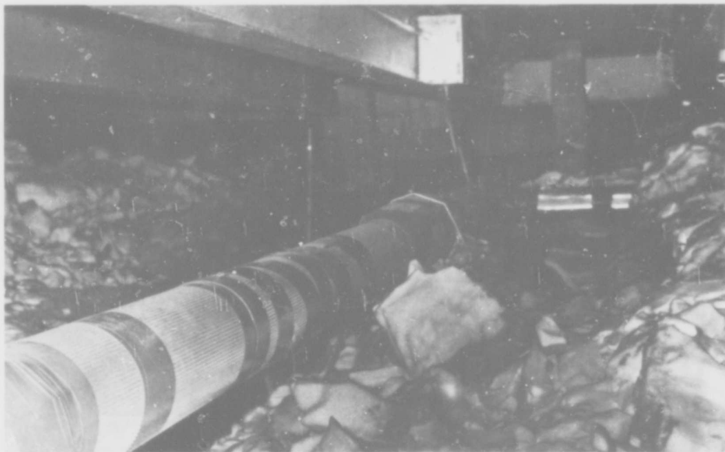
Figure 4. Utility pipes beneath Building 155 that required extensive digging to provide access for repair.
