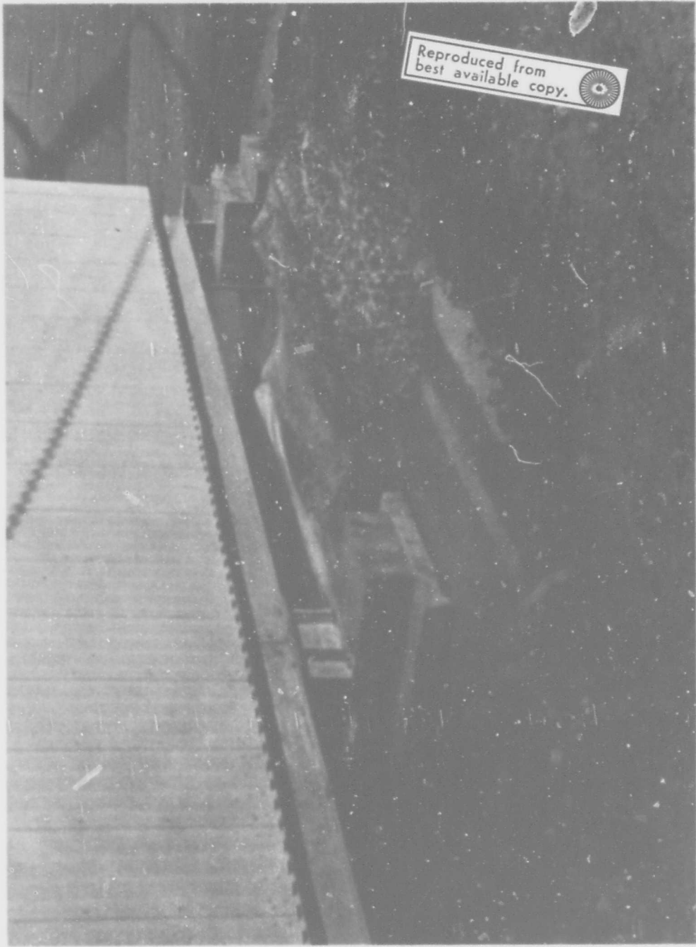
Figure 5. Melt water around footings of Building 155.
