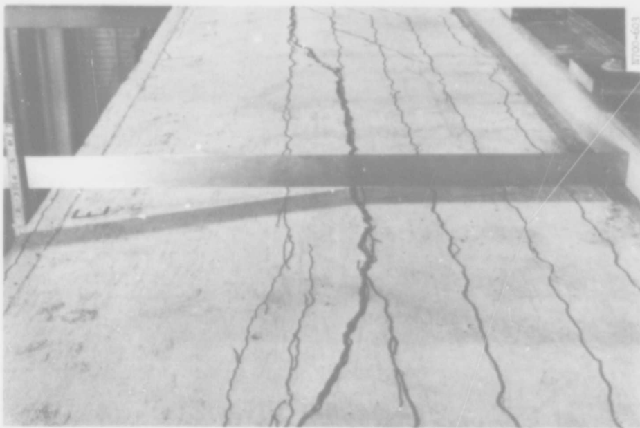
Figure 4.29 Rotation at east wall midheight after Dynamic Test II.
