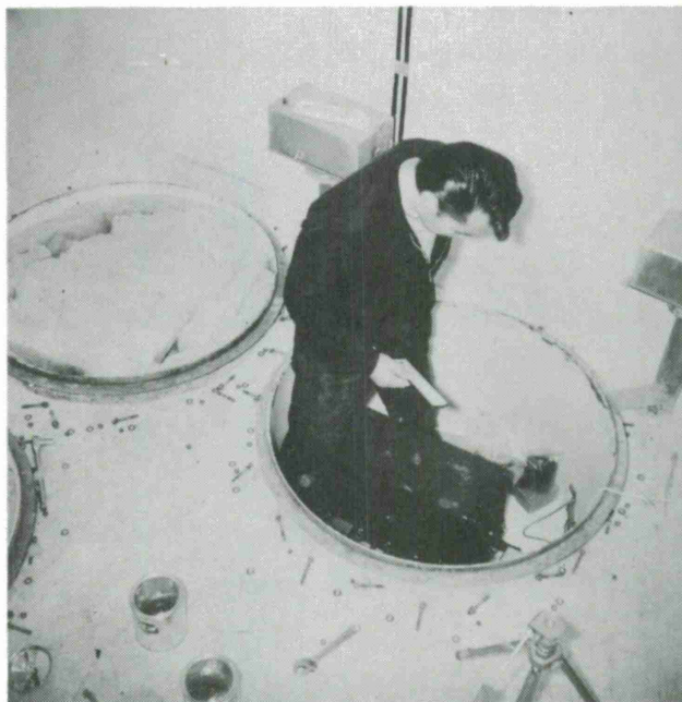
Figure 3.1 The NS and the EW tanks opened, the NS tank with insulating pads in.
