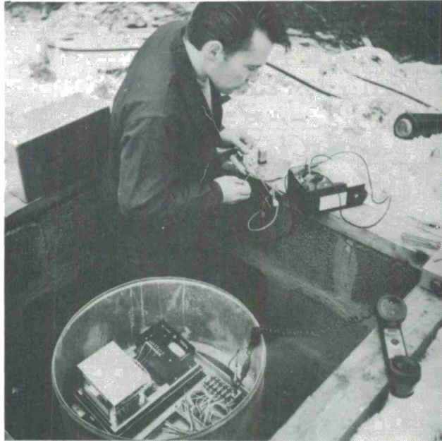
Figure 4.3 Technician adjusting damping resistor at the WHV.
