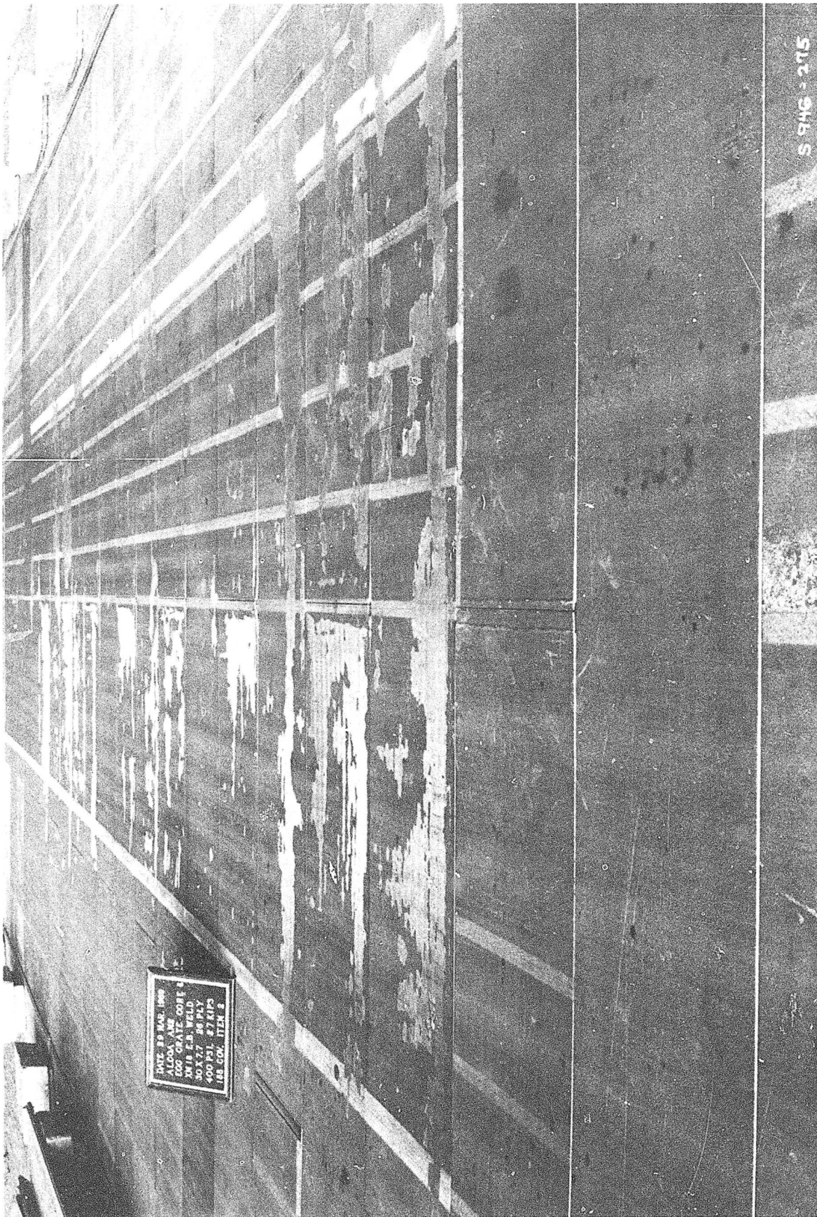
Photograph 14. Item 2 at failure after 188 coverages
