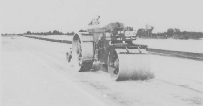
Fig. 2. Using steel-wheel roller to roll out ruts in soil subgrade beneath membrane surfacing
