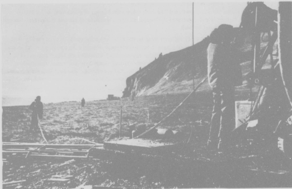
Figure 7. Inserting the three 1000-ft thermistor cables in hole C. The cables were laid out on the ground and "walked" in by six men.
