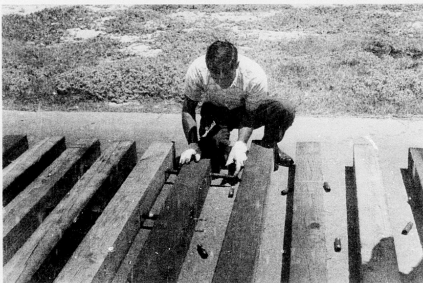
Figure 6. Prototype flexible timber ramp being assembled using 4-inch long pipe nipples as spacers.
