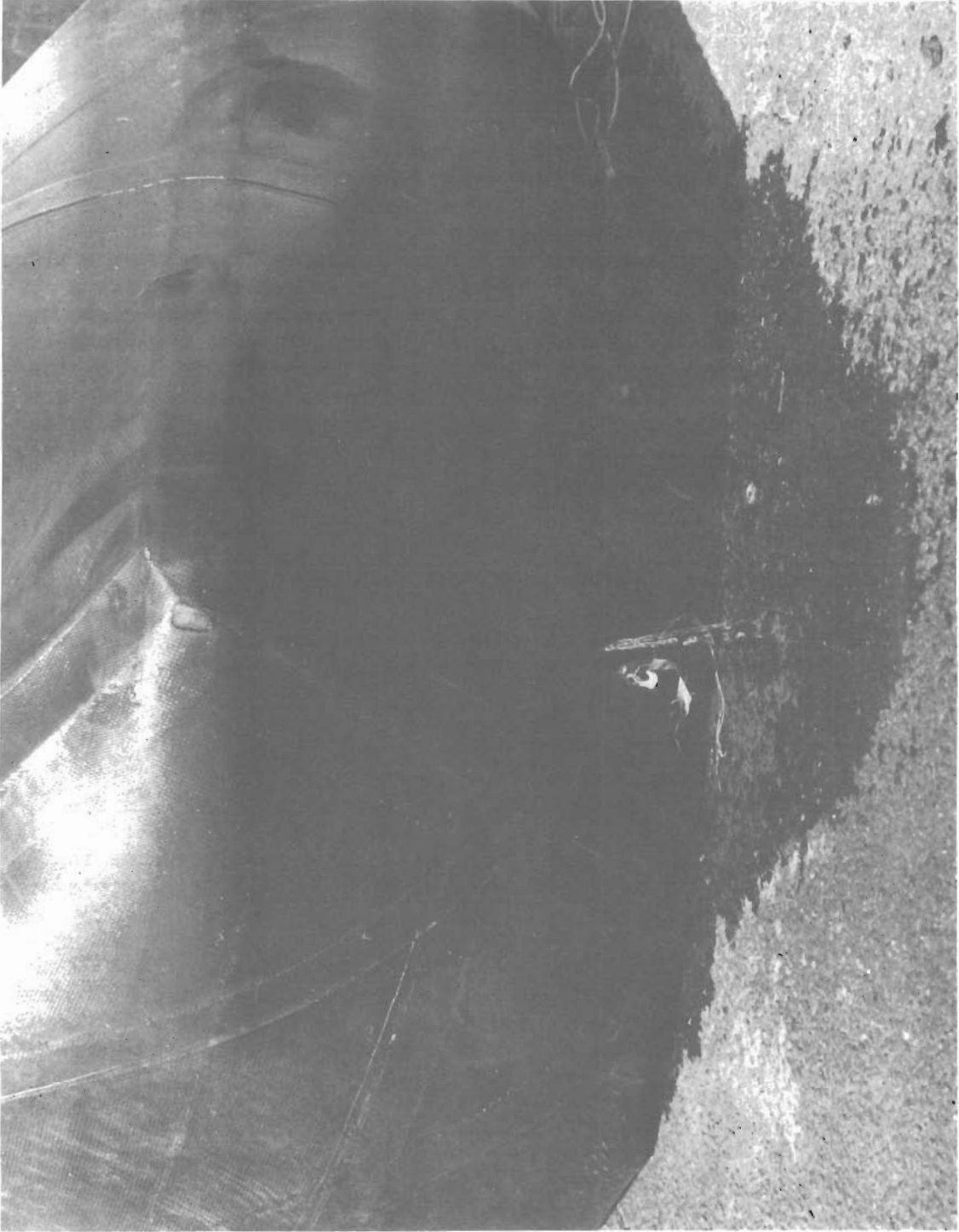
Figure 26. Close-up of Cut and Leakage.
