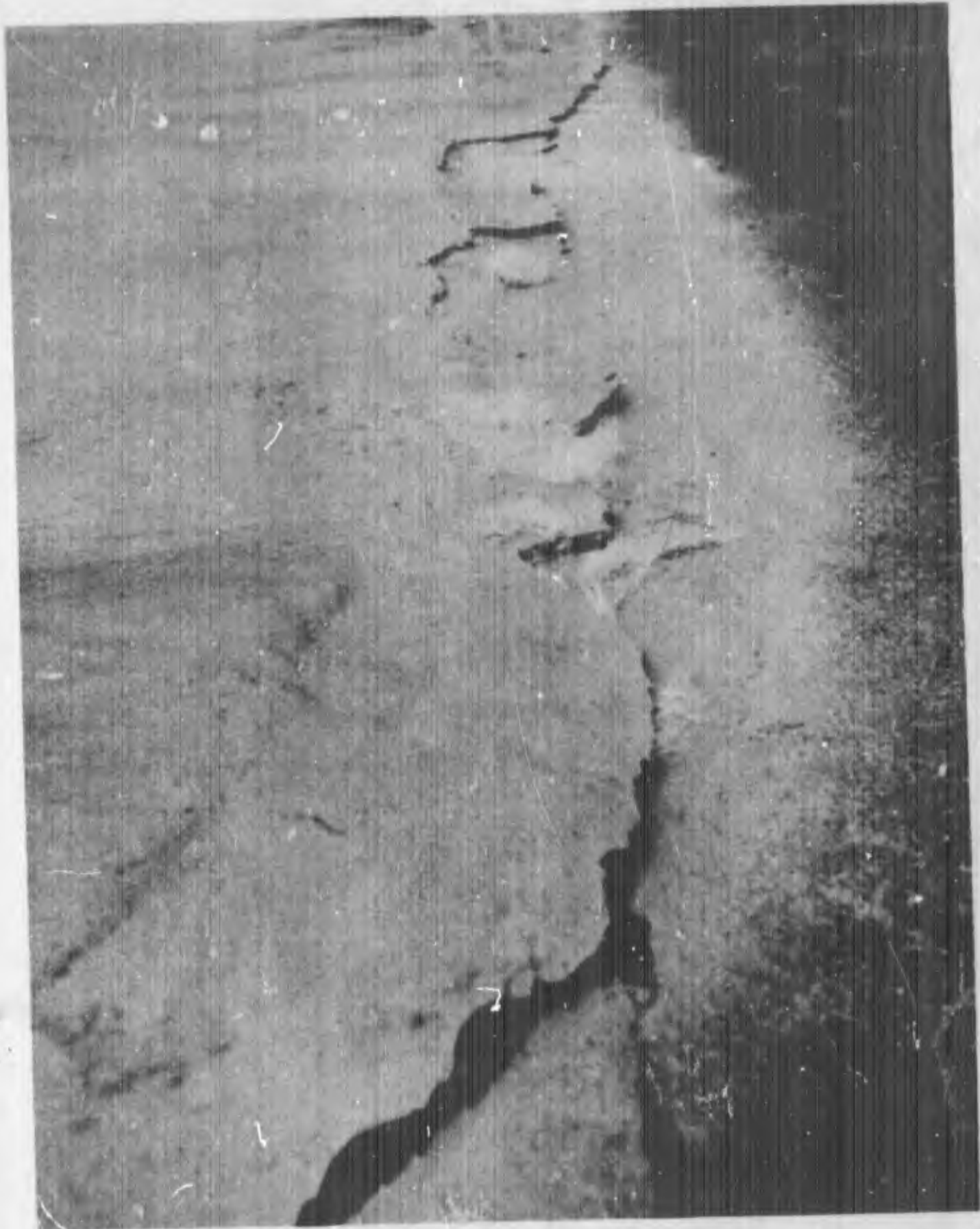
Figure 156. Runway Side Crack, German Pad.
