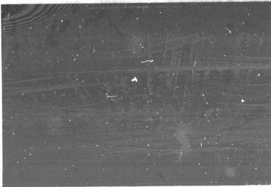
Figure 6. Lane 18, general view showing transverse straightedge measurement at 30 coverages (failure)
