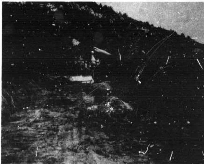
Figure 21. Road building in area of Z9 showing terrain typical of the lower brush country at TFSO
