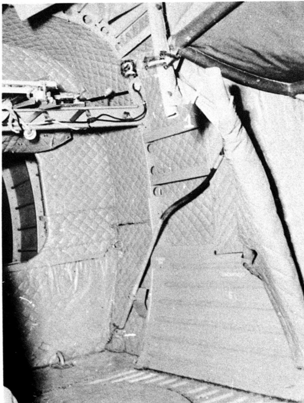
Fig. 25. View showing failure of luggage compartment post (arrow 1) at the attachment point of seat 4L. The attachment bracket is indicated by arrow 2.
