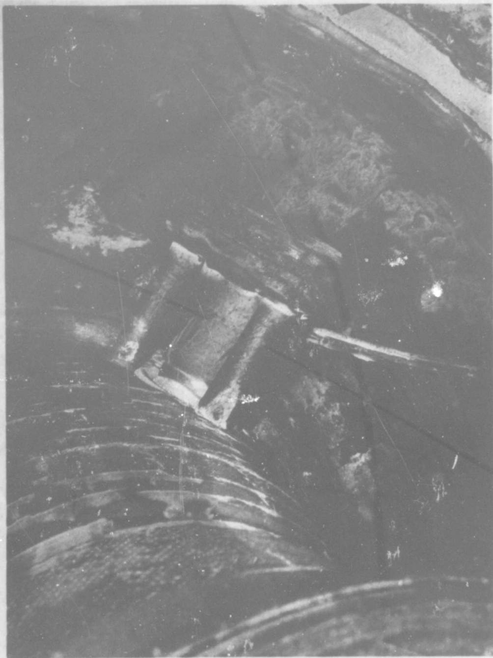
Figure 11. Valve 1 After Test
