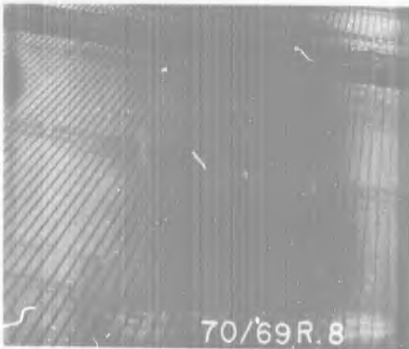
Fig. 17. Grooving at transverse crack in continuously reinforced pavement.
