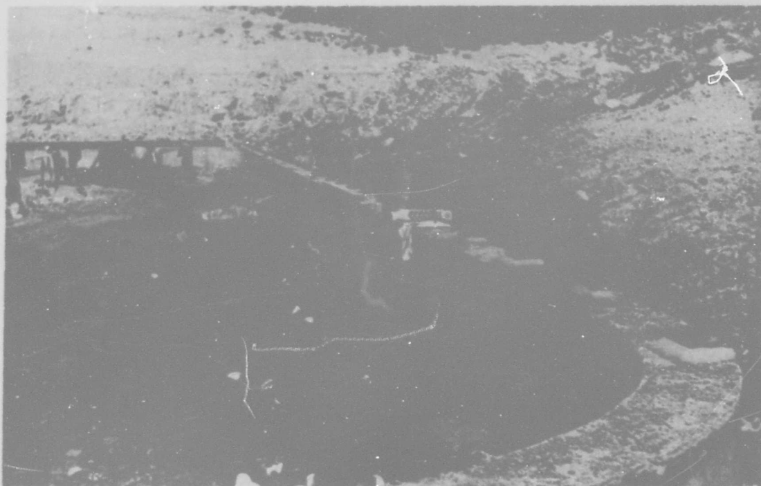
Figure II-12. Concrete Perimeter Walls, Anchor Bolts and Leveling Plates.
