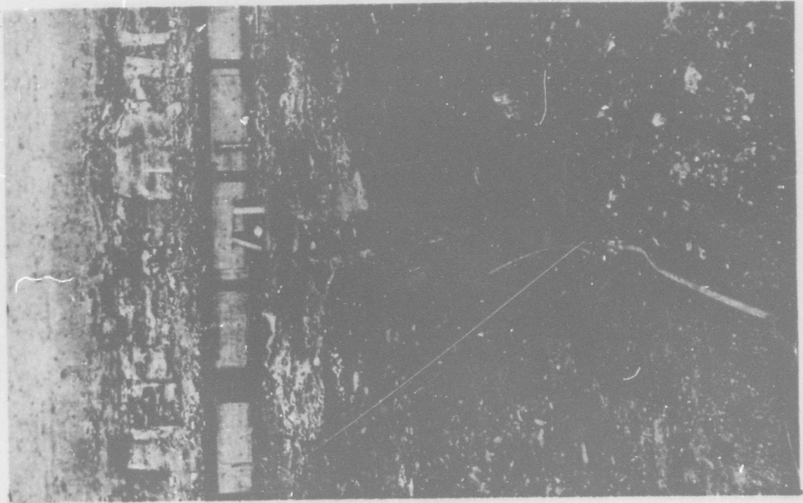
Figure II-22. Jack-hammering for Instrumentation System. (Results of pre-splitting attempt shown beyond construction worker).
