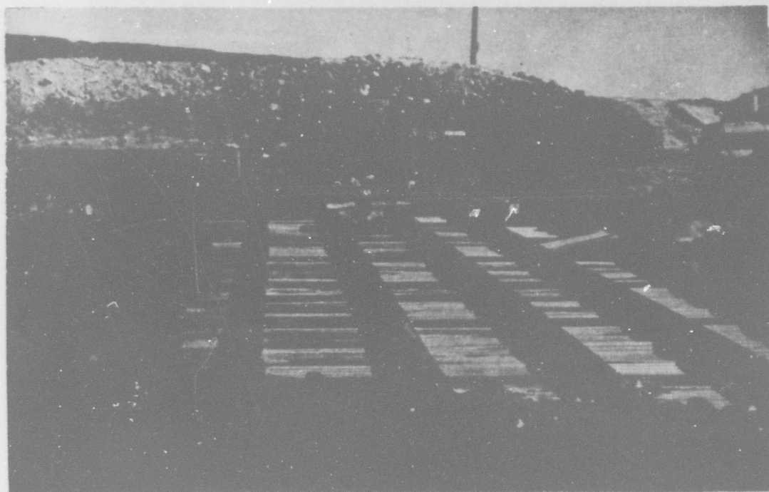
Figure II-86. Overpressure Structure Showing Subdeck and Subdeck Earth Fill Prior to Placing Roofdeck on Top of Wide Flange Beams.
