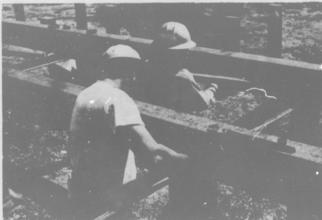
Figure II-84. Erection of Structural Steel for Overpressure Structure Showing Installation of Double Angle Struts.
