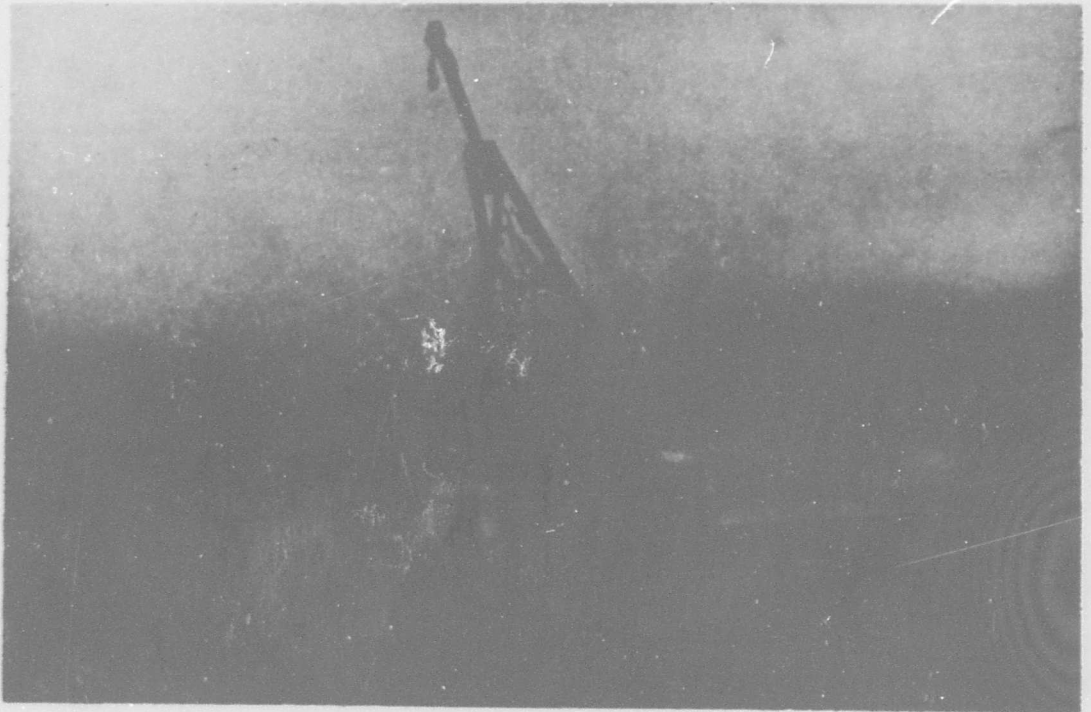
Figure II-95. Contractor Drilling Holes for Surcharge Dispersal System. Holes are 9-inch Diameter 9-feet deep.
