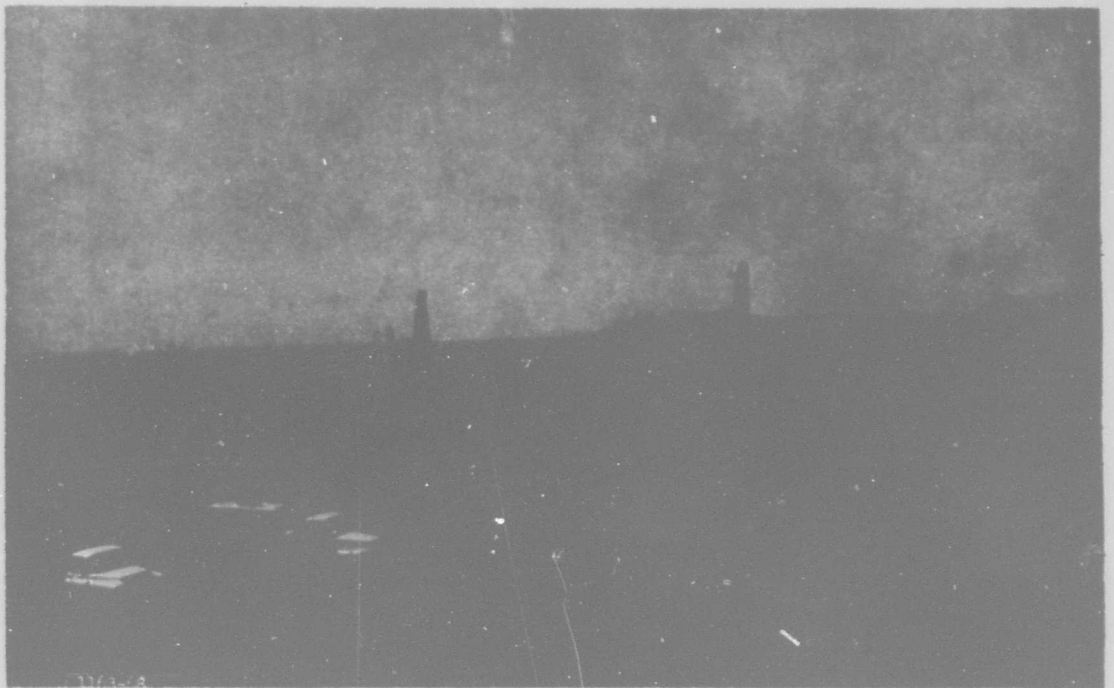
Figure II-3. Test Site in Early Stages Showing Corps of Engineers Drilling Rigs and Contractor's Equipment.
